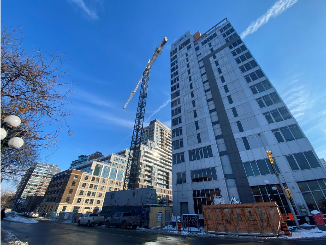
Image showing the subject property at 110-116 York Street looking south east, with the existing hotel building at the corner (right) and development project next door at 126 York Street.
