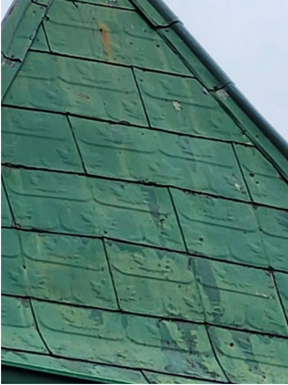
Close up of tin pyramid roof with maple leaf pattern detail. (Source: City of Ottawa, 2025.)
