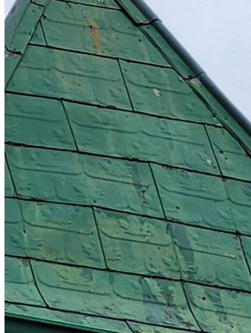
Close up of tin pyramid roof with maple leaf pattern detail. Source: City of Ottawa, 2025.
