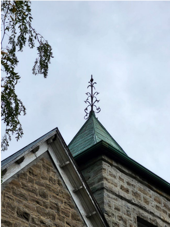
Tin pyramid roof as seen from Bank Street. (Source: City of Ottawa, 2025.)
