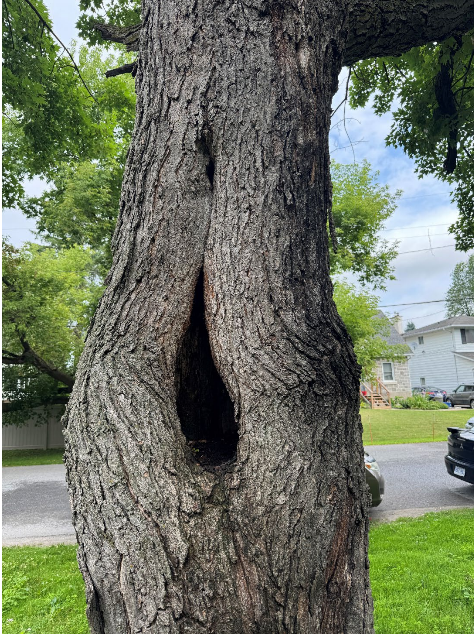
Figure 2: Cavity in the trunk of Tree 1 that likely extends to the first branch union
