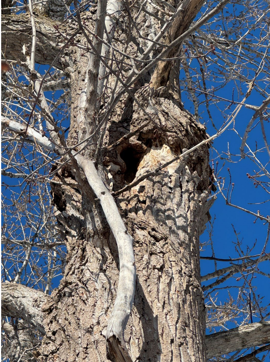
Picture 6: Large wound extending over 50% or circumference of poplar tree creating potential failure point appr 10 m up trunk
