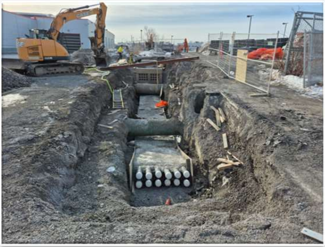
Electrical power distribution
