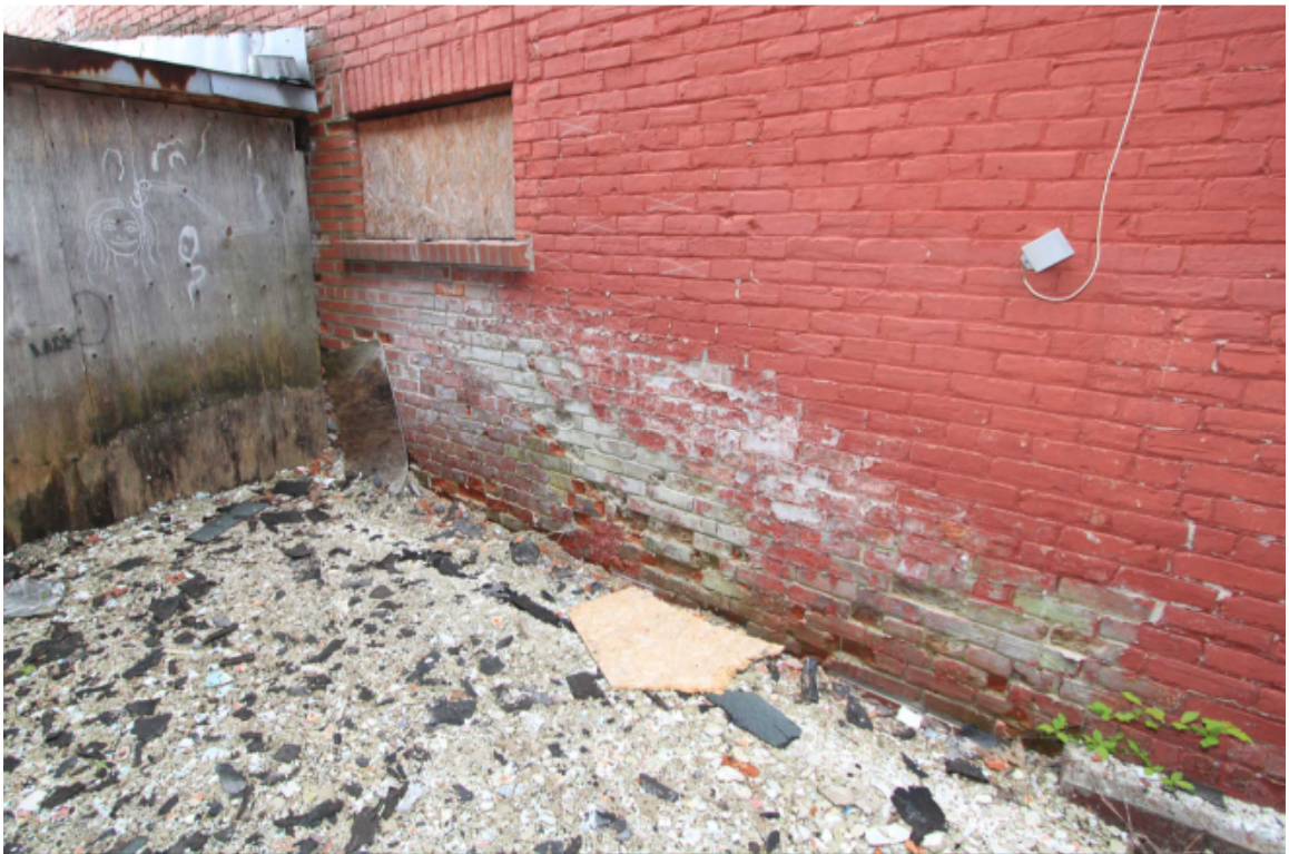
Figure 16. Frost Damage in East Wall of 197 Wilbrod Street
