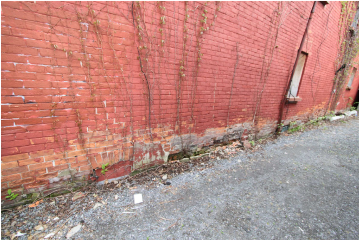
Figure 17. Frost Damage in East wall of 201 Wilbrod Street
