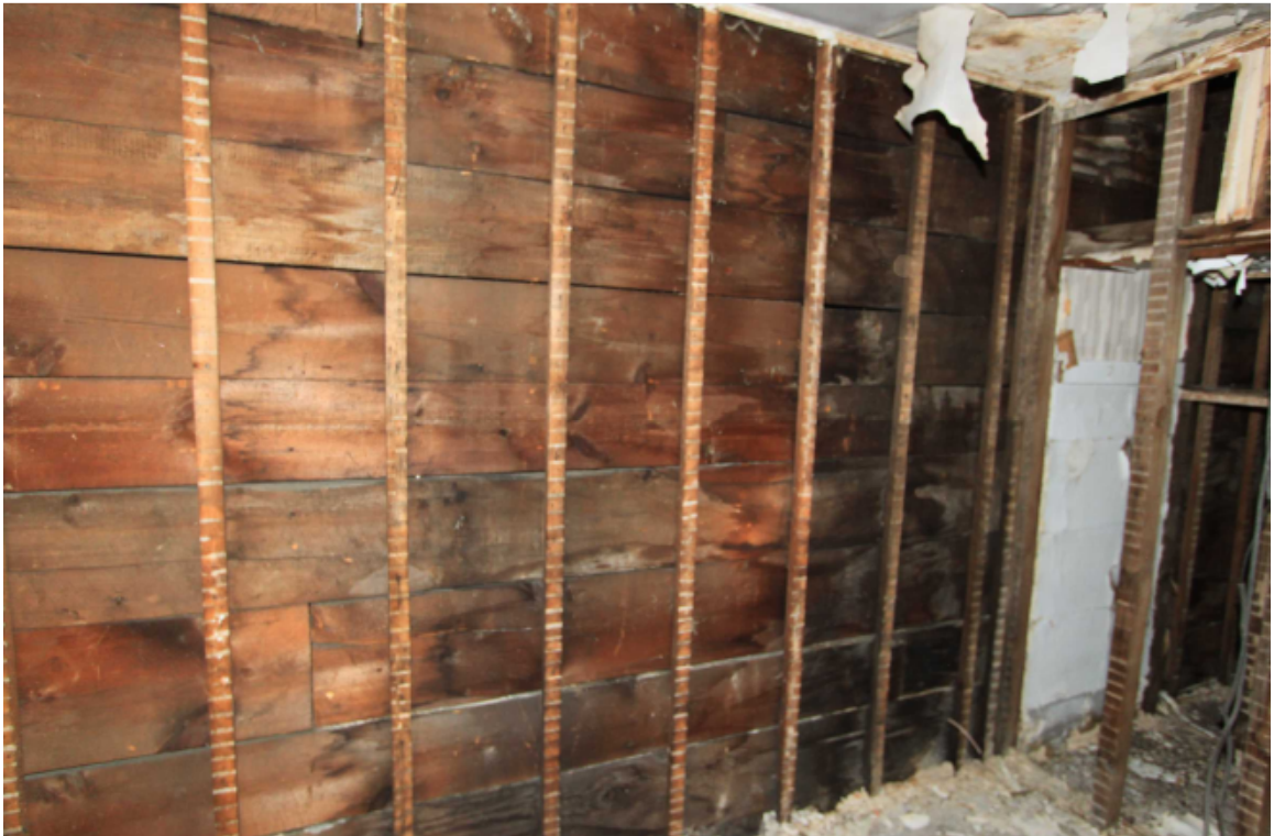
Figure 10. Water Staining of Exterior Walls
