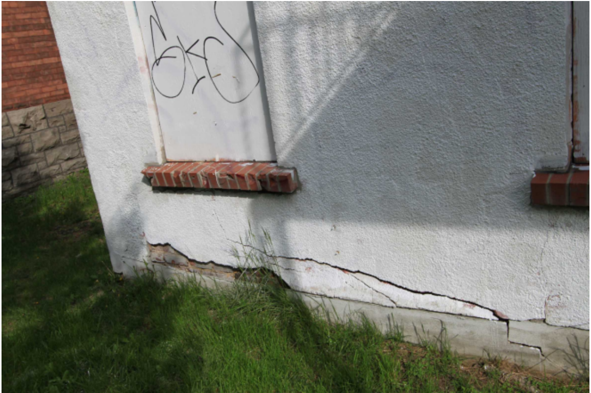
Figure 15. Close-up of Deteriorated Stucco and Brick Behind
