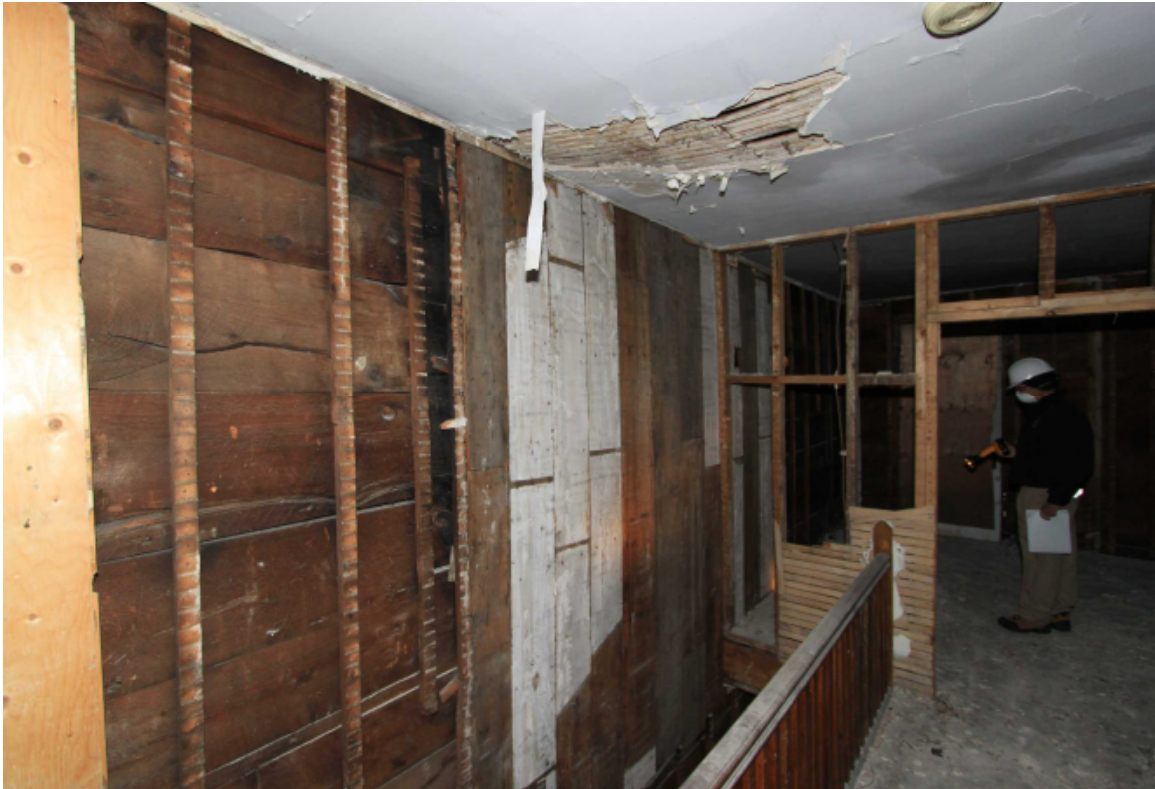
Figure 12. Fire Damage Repaired with Vertical Planks
