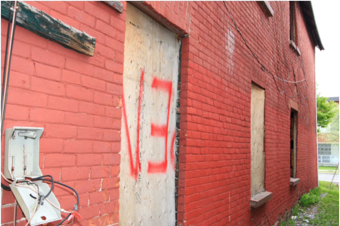
Figure 13. Bulged Brick Veneer - West Wall of 197 Wilbrod Street
