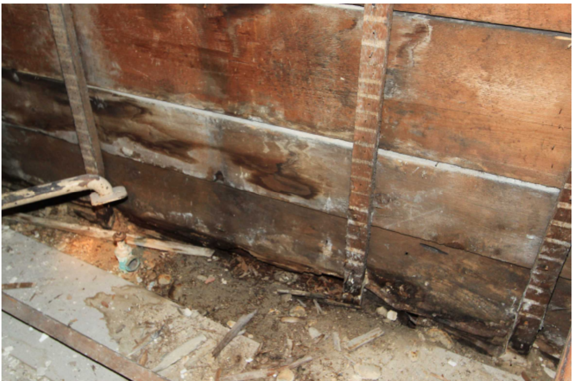
Figure 11. Deteriorated Plank at the Base of Wall
