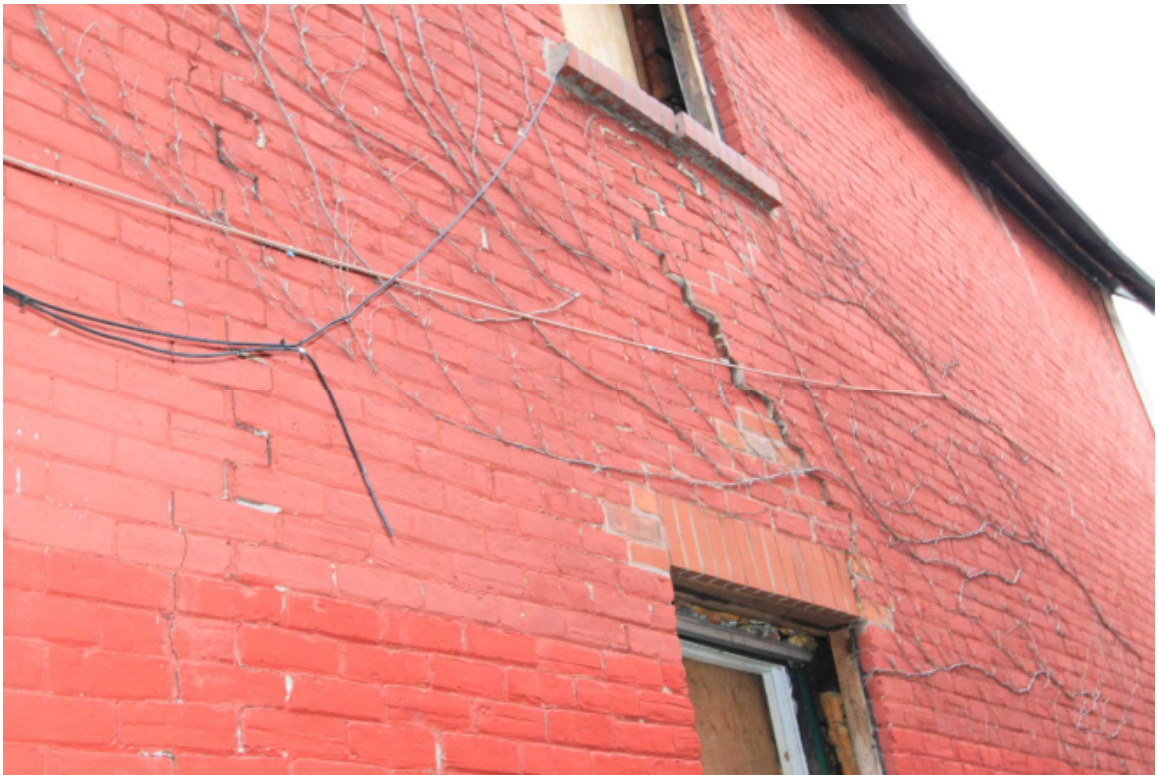
Figure 14. Close-up of Large Crack at the Bulge
