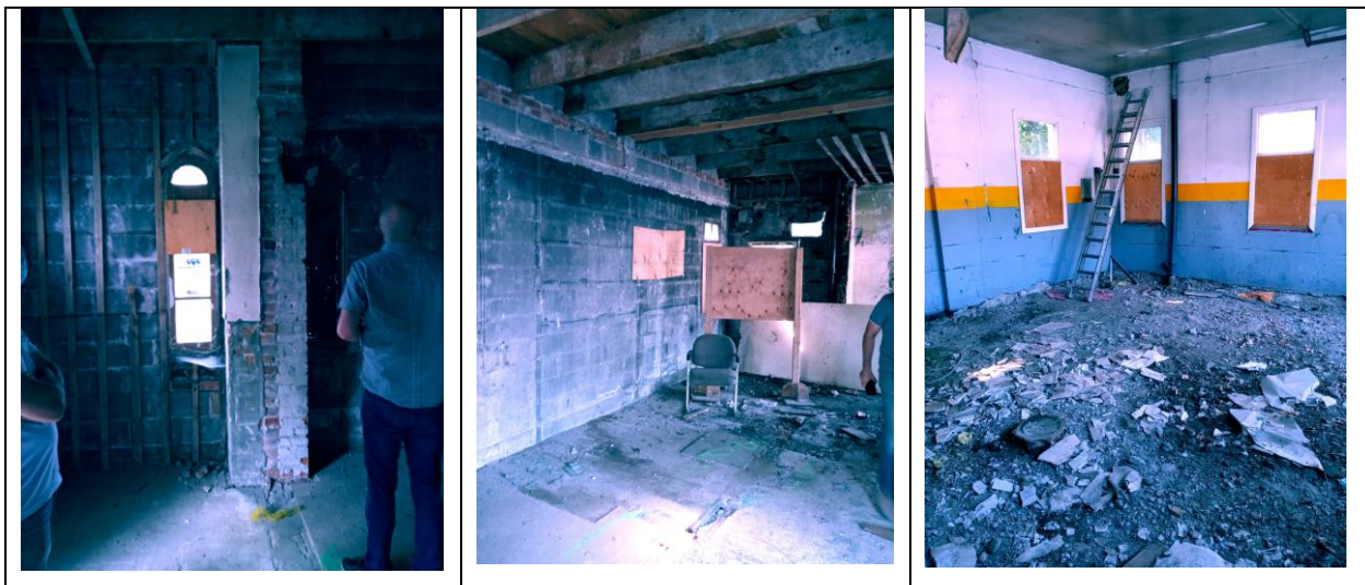
Figure 6: Interior views illustrating the condition, with the interior stripped down to the block walls.
