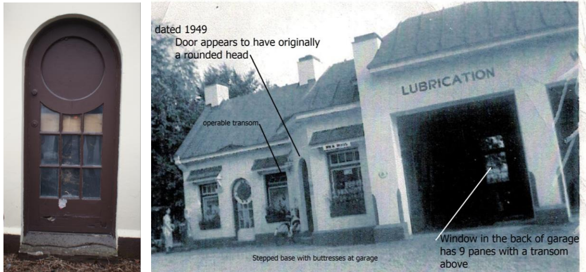
Figure 9 : Circa 1949 – 50. The historic view of the Service Station provides reference information supporting the conservation of the round headed doors at both entrances. Other features include the stepped foundation with chamfered treatment at the base of the service bay entrances. Over time, the scale of the stepped foundation has been reduced as grade was raised with the addition of asphalt. Source: Ottawa Archives, John Newcomb Collection.
