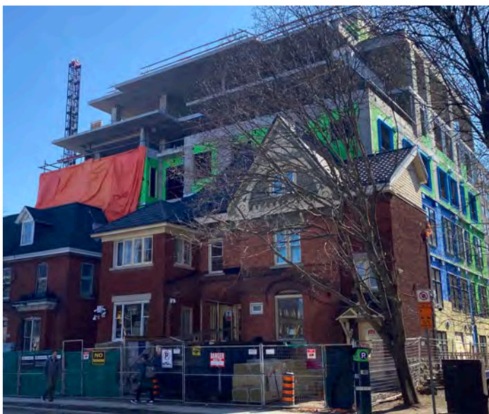
Figure 25: This project once complete will incorporate two contributing historic buildings into a larger apartment building behind.
