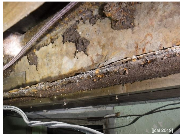
Figure 4: Corroded Beam at Basement
