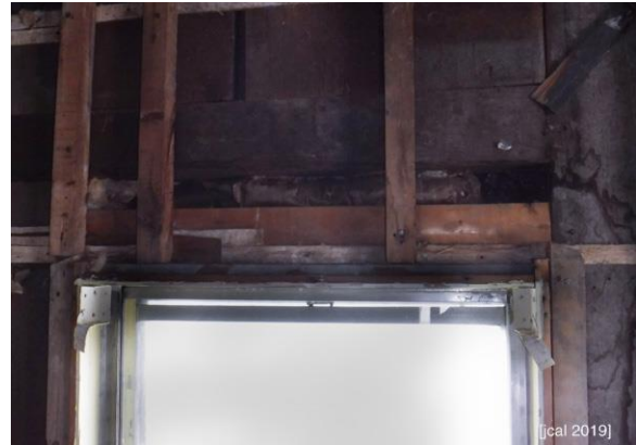
Figure 2: Rough Opening at Window, note unfilled space above
