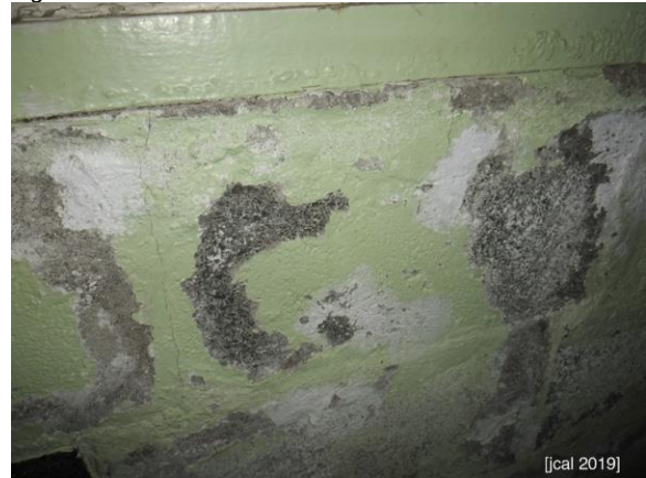
Figure 10: CMU Foundation Wall Condition
