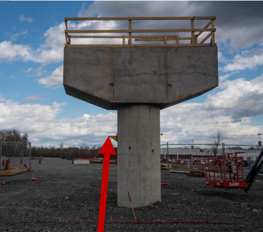
Infrastructure (est) de la promenade Uplands
