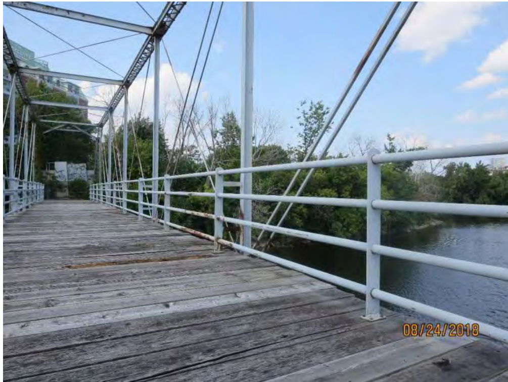
Photograph 25: Typical condition of hand rails and posts.
