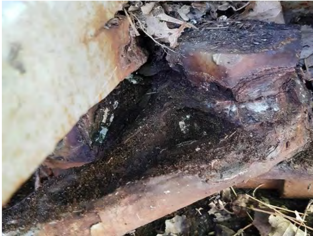
Photograph 35: Severe (> 25%) section loss of cross brace at South Abutment.
