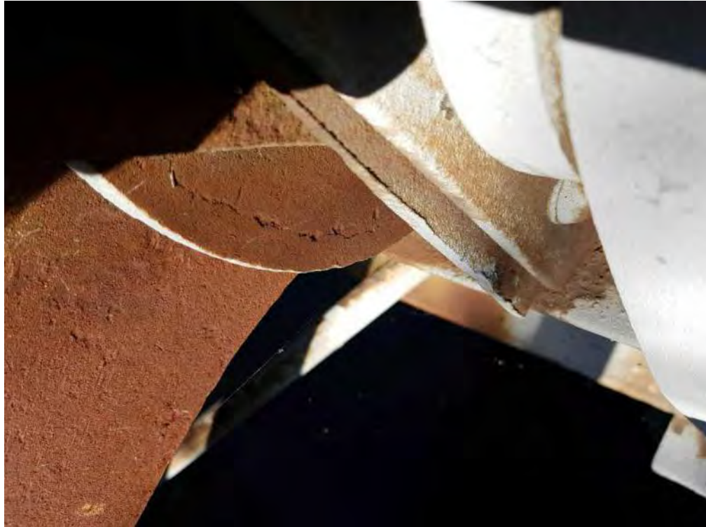
Photograph 17: Typical surface defect on bottom chord members at pin connections.
