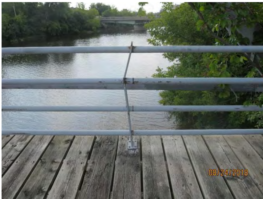
Photograph 26: Deformed post near North Abutment.
