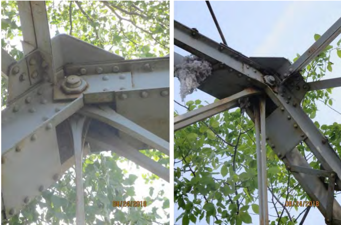
Photograph 7: Typical top chord to end post connection. Debris/nesting was noted at southeast corner of the structure.
