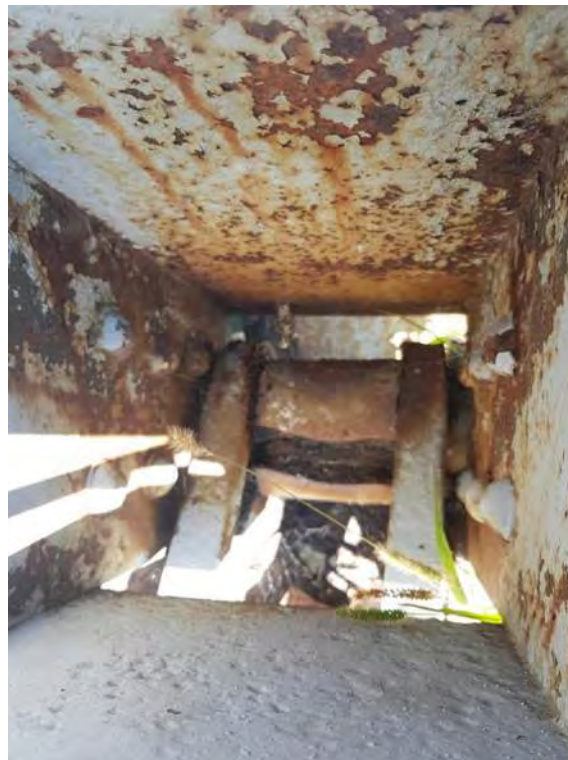
Photograph 40: Cracked and corroded spacer on southwest pin at Pier.
