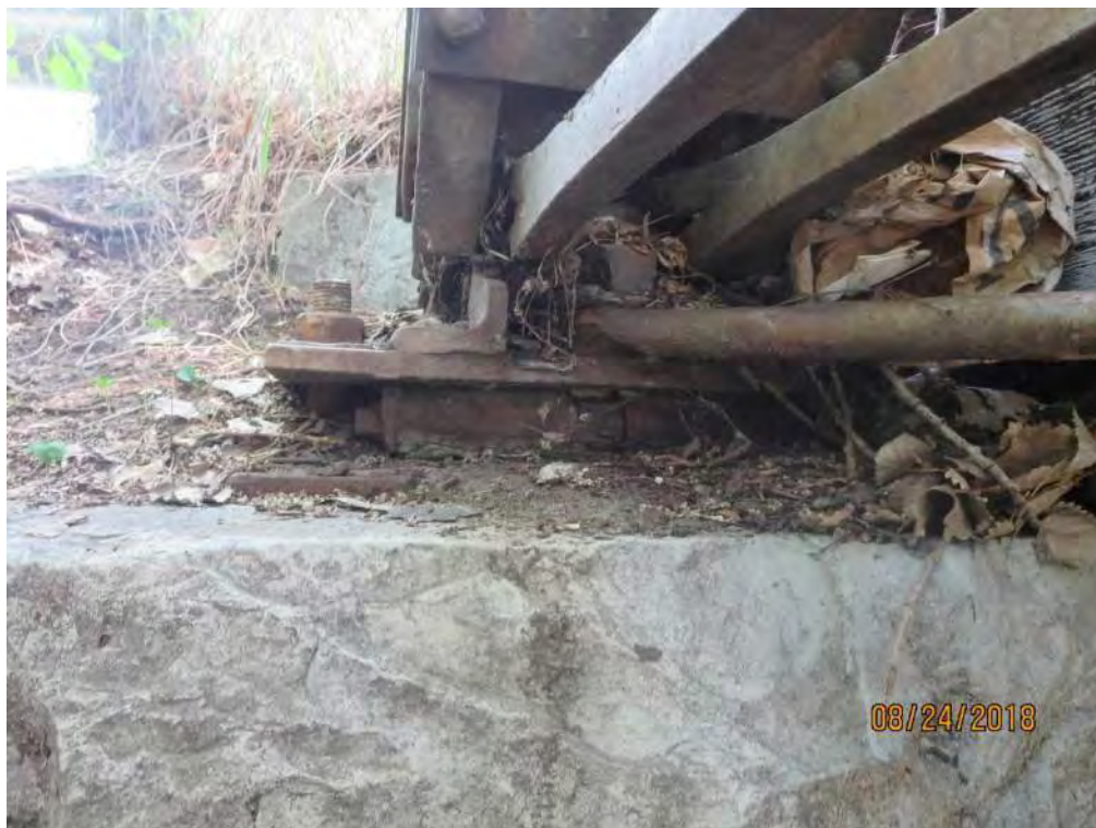
Photograph 36: Typical abutment roller bearing. Southeast bearing shown. Bearings are suspected to be seized.
