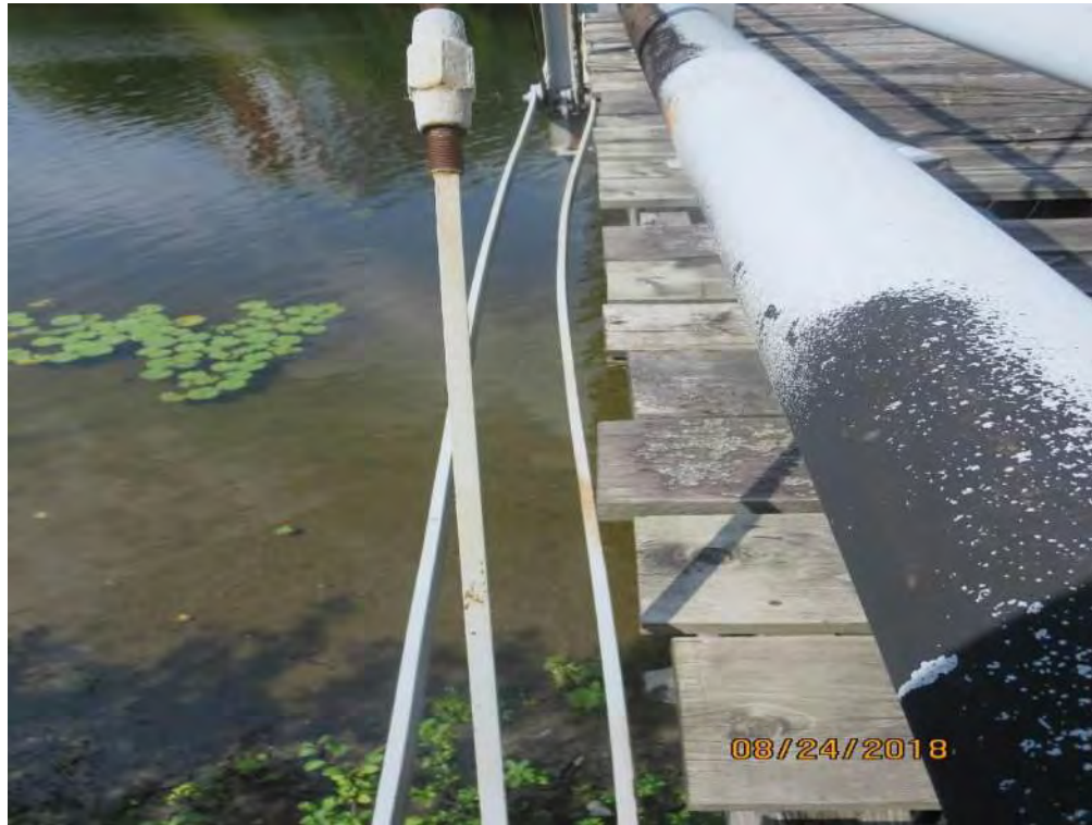
Photograph 19: Bowed and disengaged bottom chord at an interior truss panel. This deformation was observed at several locations.
