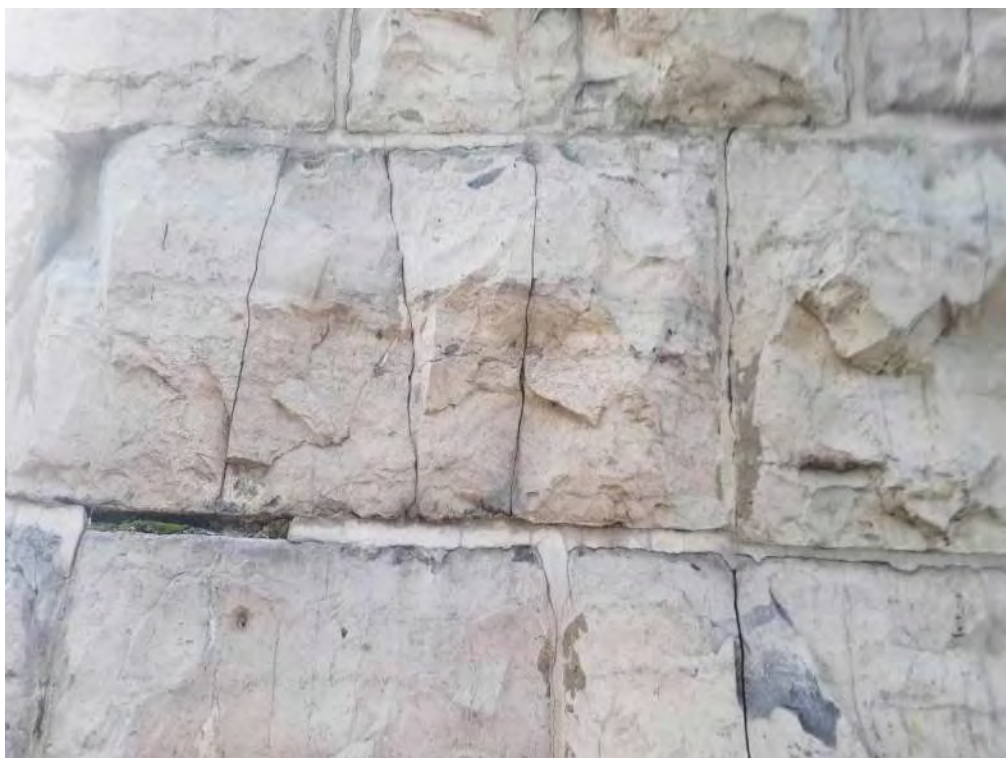
Photograph 48: Vertical cracks and loss of mortar at Pier.
