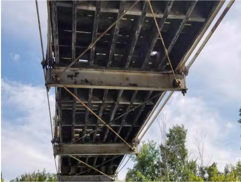
Photograph 31: Typical condition of floor beams. Floor beams generally in fair to good condition with corrosion typically limited to deck curb line and localized coating failure (peeling, light to severe surface rust).
