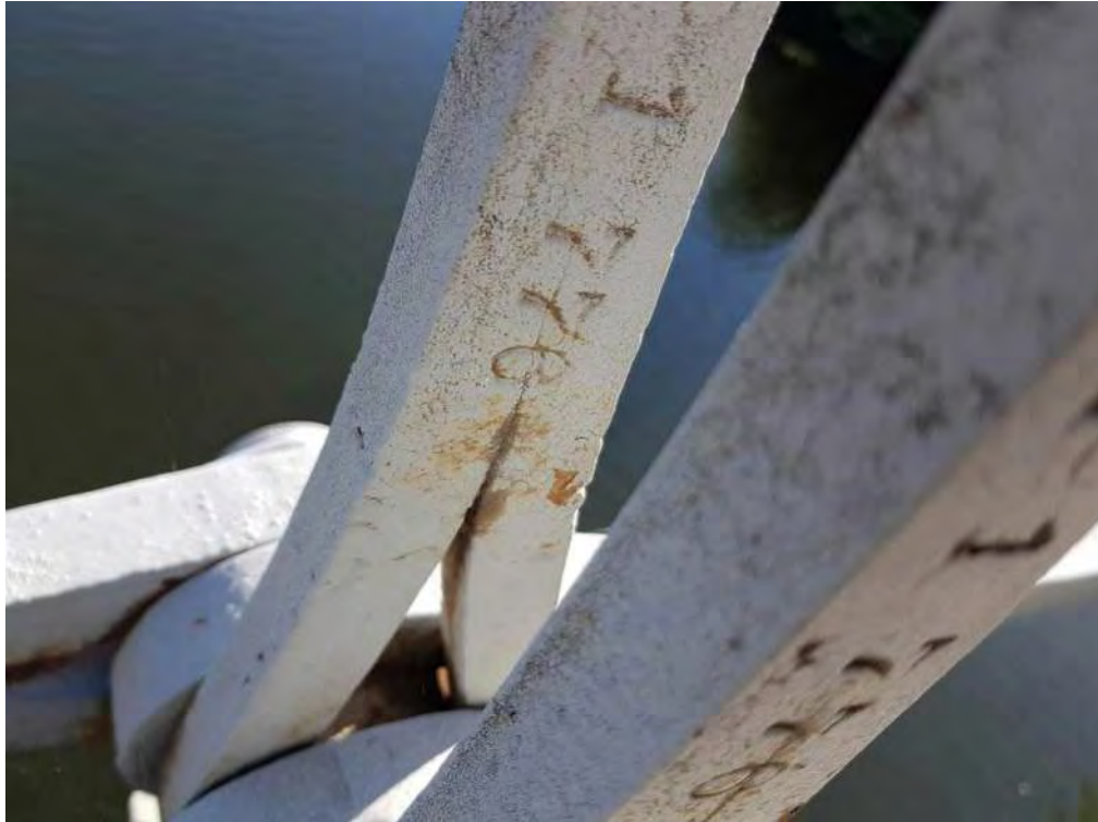
Photograph 13: Possible crack initiation at loop welded forged eye bar. Typical condition noted at several eye bar locations for verticals and diagonals.
