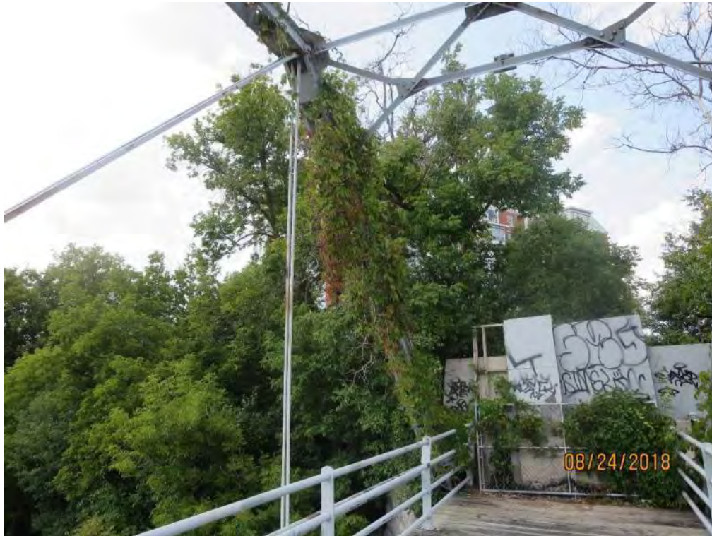
Photograph 9: North end of structure with blocked access. Note vegetation on end post.
