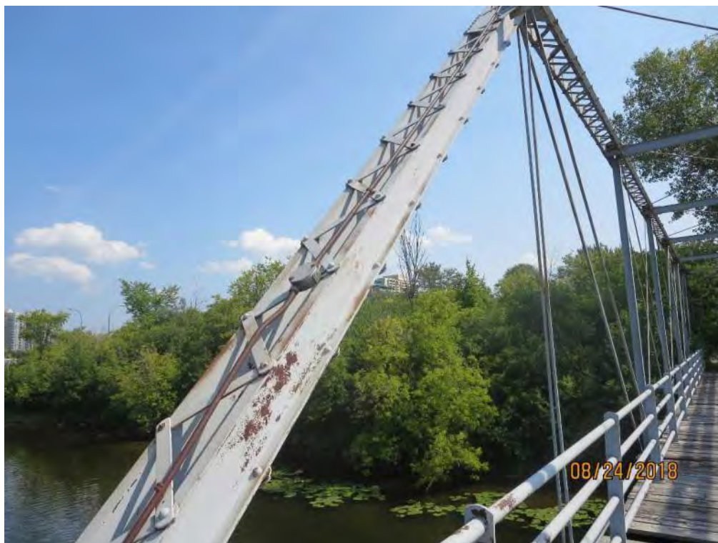
Photograph 6: Typical condition of end post.
