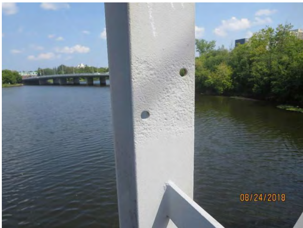
Photograph 10: Typically pitting corrosion on truss verticals at previous railing connection.
