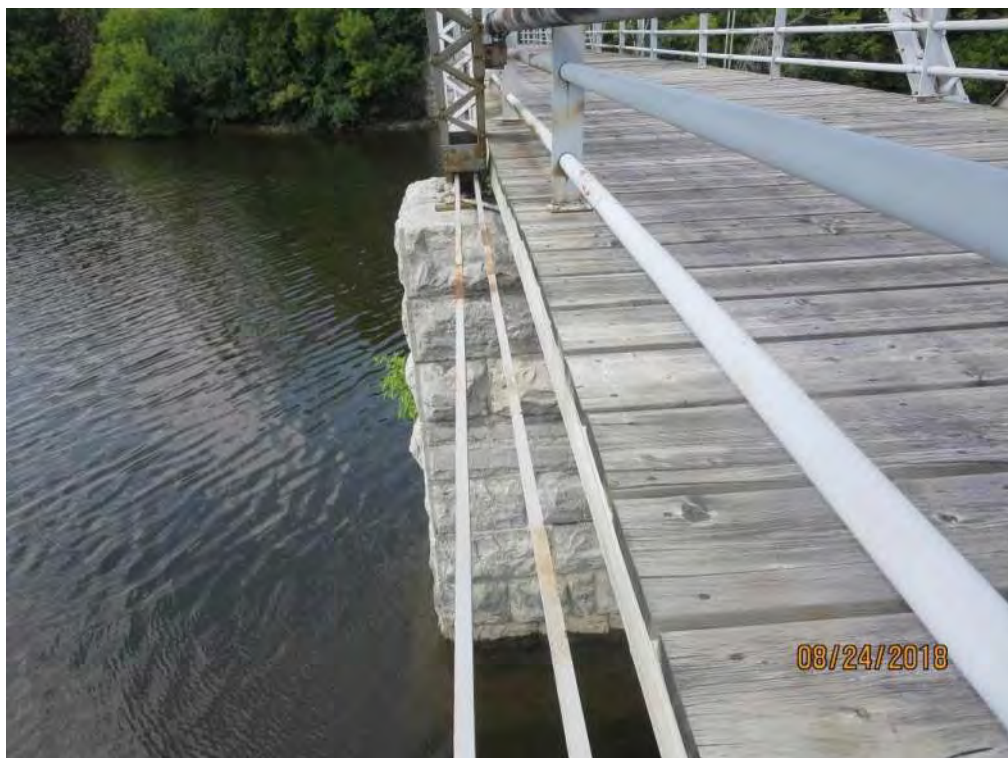
Photograph 18: End panel square rod bottom chord members within south span at pier. The bottom chord appeared engaged at this location.
