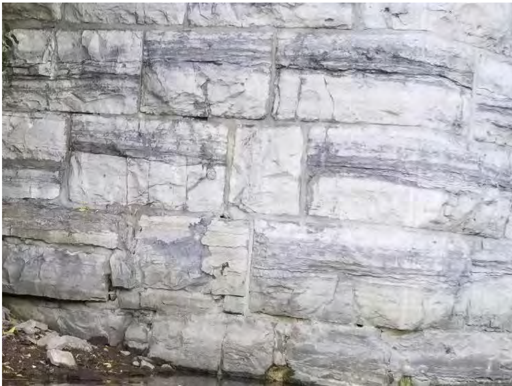
Photograph 44: Close up of the west wingwall showing some vertical cracks and localized spalling of stone.
