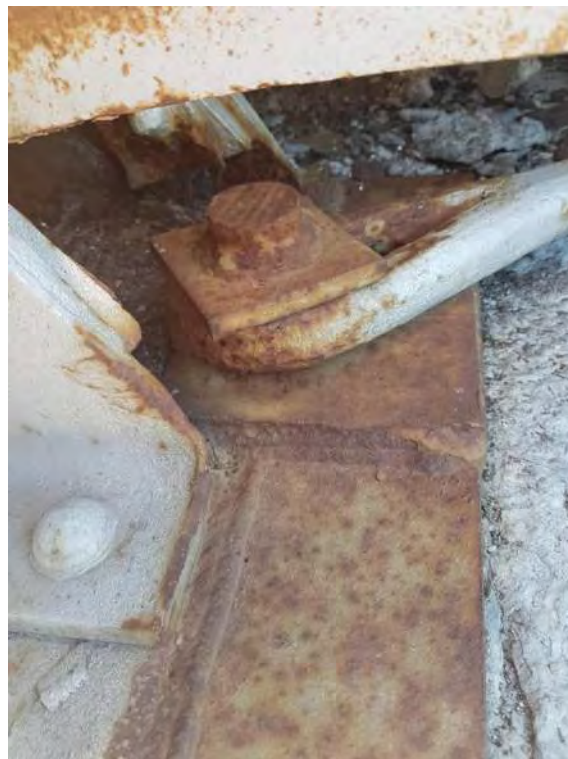
Photograph 34: Evidence of retrofit due to welded plate connecting cross brace to bearing plate and pier.
