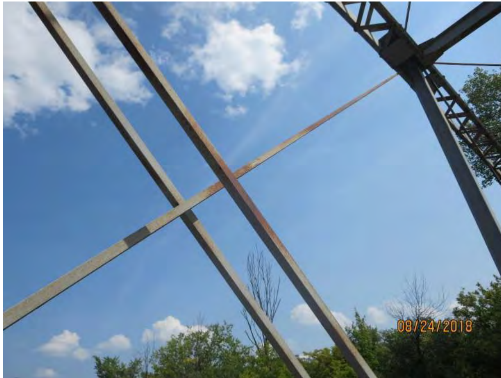
Photograph 11: Typical configuration and condition of diagonals.
