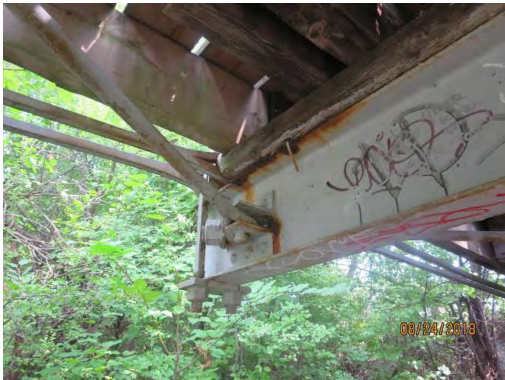
Photograph 32: Typical corrosion of top flange at floor beam ends (below curb line).
