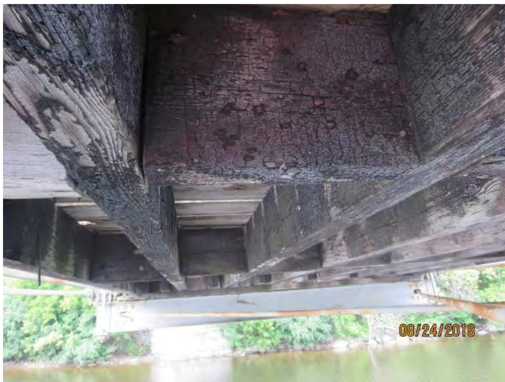
Photograph 30: Light to medium fire damage to stringers and blocking near South Abutment.
