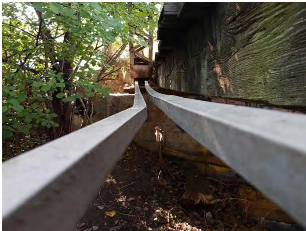
Photograph 20: Deformed / disengaged bottom chord at end panel near South Abutment.
