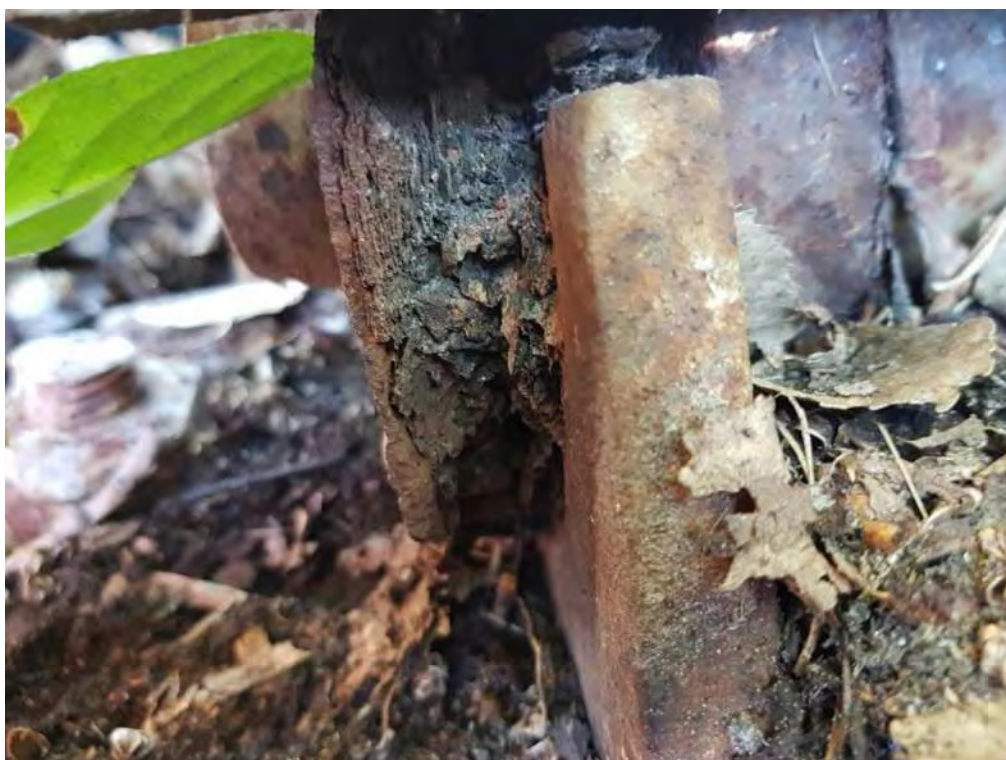
Photograph 38: Severe corrosion and rust jacking of end post at South Abutment pin connection.
