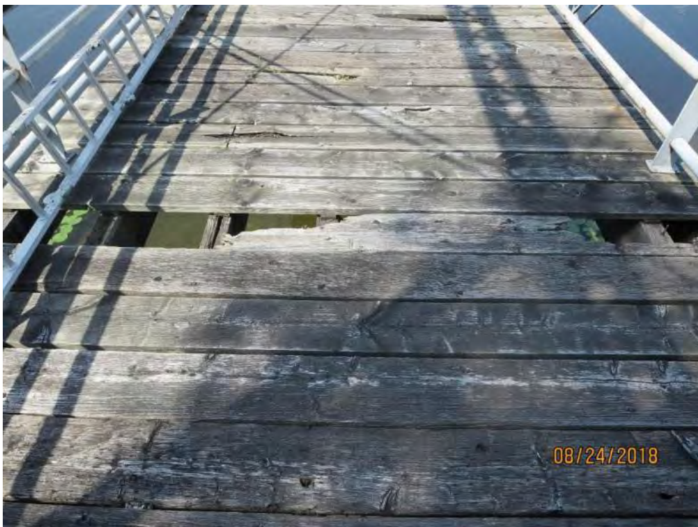
Photograph 24: Close up of deck condition. Note that several planks are damaged, severely weathered and rotting.
