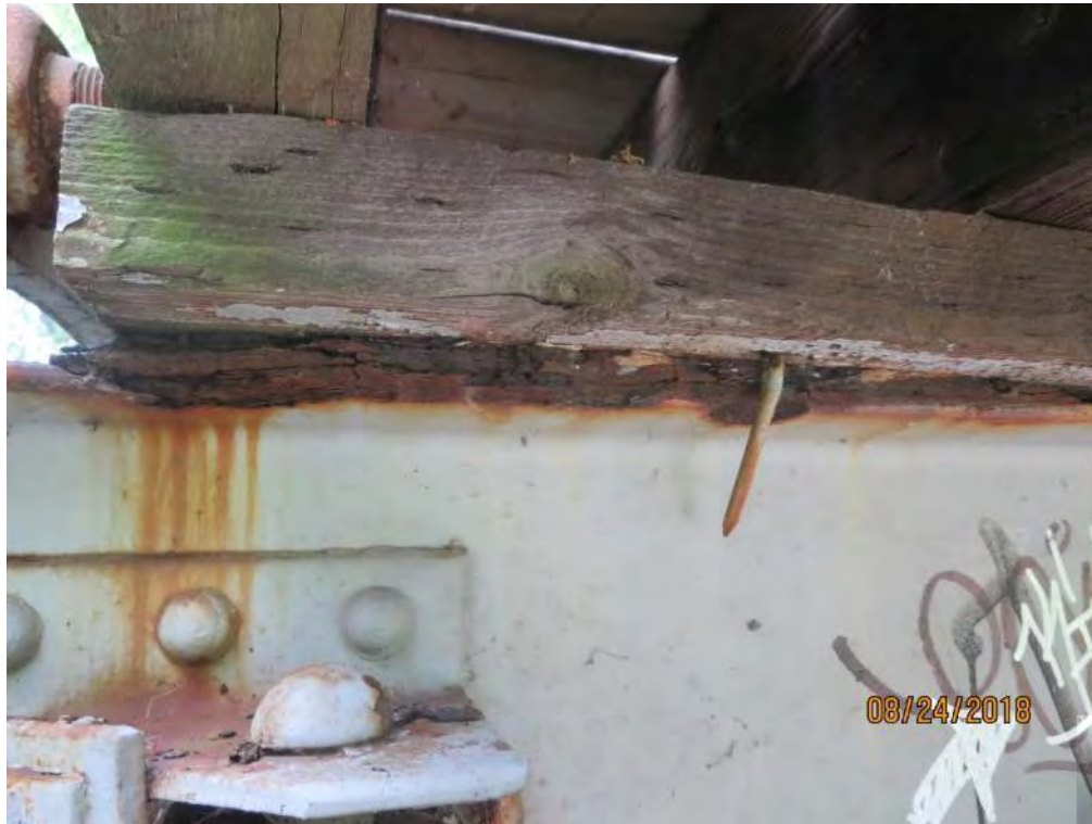
Photograph 33: Close up of Photograph 34, showing severe corrosion and perforation of floor beam top flange near South Abutment.
