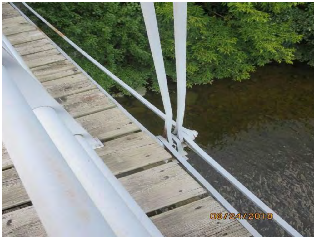
Photograph 12: Kinked exterior vertical at north end of north span.
