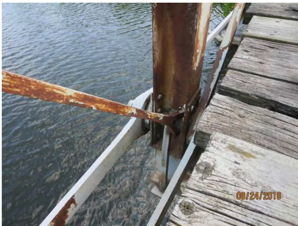
Photograph 16: Severe flaking of coating on interior panel vertical at middle of North span.
