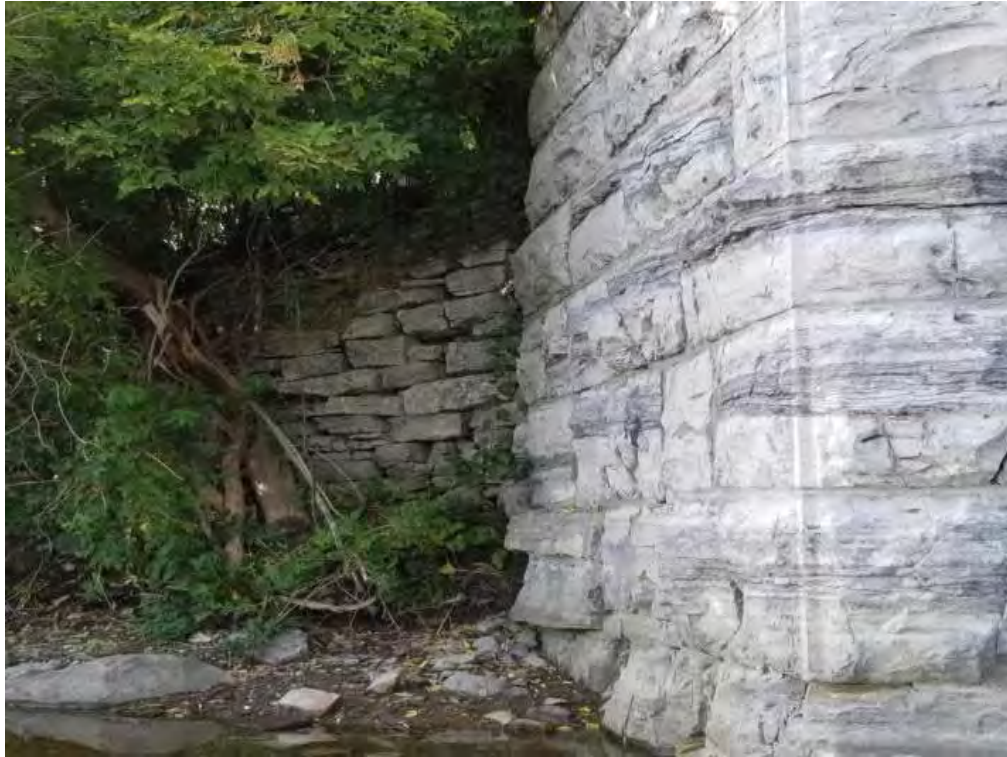
Photograph 43: West wingwall and dry stone masonry retaining wall at the North Abutment.
