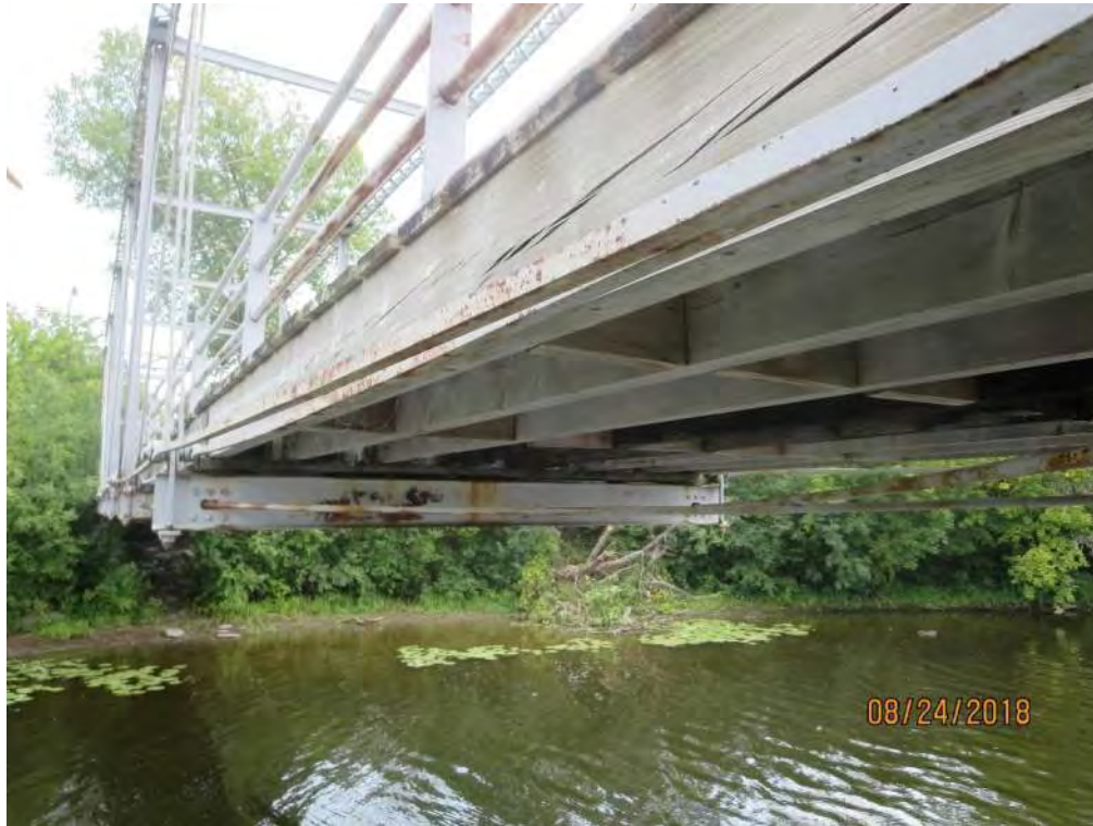
Photograph 27: Light to medium checking and splitting of replaced outer stringers (typical condition).
