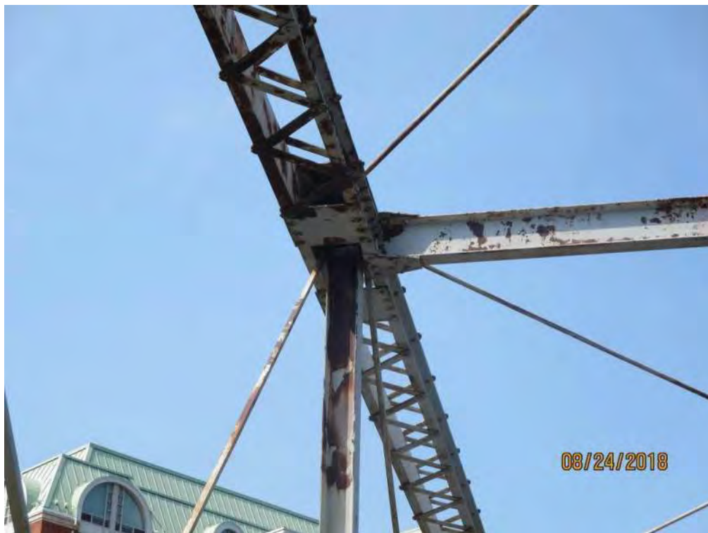
Photograph 8: Interior vertical and brace configuration. Coating failure noted at this connection (north span).
