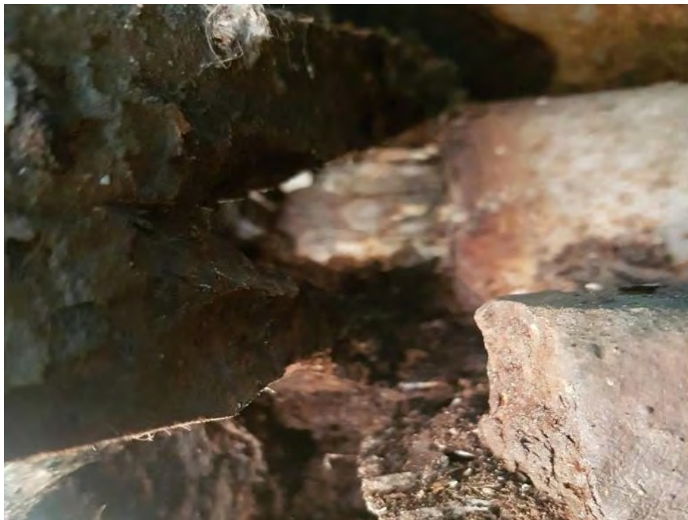
Photograph 22: Close up of Photograph 21. Note approximately 50% section loss of one of the rods.
