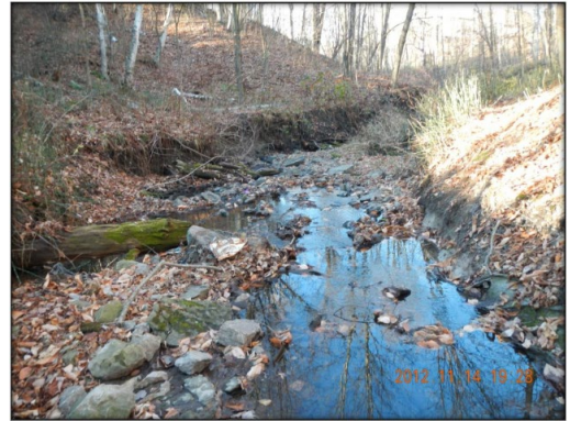
Photo 26: Erosion site #3 along Reach VC-9
