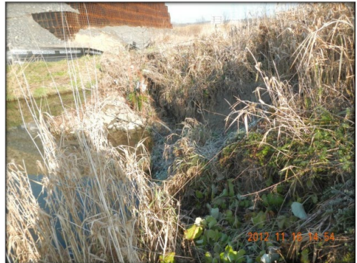
Photo 30: Erosion site #2 along Reach MEC-1
