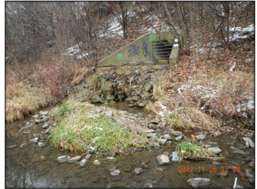
Photo 28: Erosion site #4 along Reach CD-3
