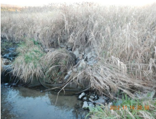
Photo 31: Erosion Site #4 along Reach TC-1B
