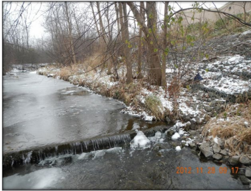
Photo 27: Erosion site #2 along Reach CD-1
