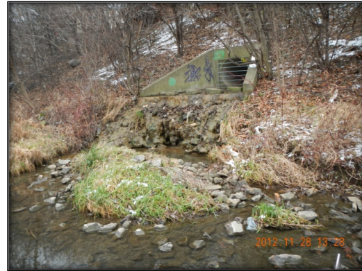
Photo 16: Priority Erosion Site Along Cyrville Drain Consisting Of ~2.0m Drop To Channel Bed Due To A Broken Storm Sewer Outlet Structure.
