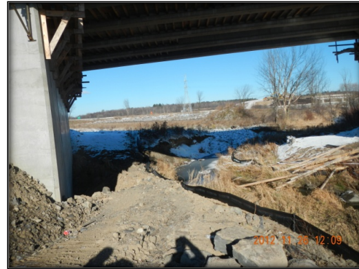
Photo 18: Priority Erosion Site Along Mather Award Drain Due To Steep Banks Identified At Newly Constructed Road Bridge.
