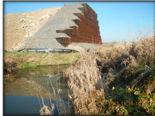
Photo 20: Priority Erosion Site Along McEwan Creek Due To Steep Banks And Slumped Material Identified Upstream Of Newly Constructed Road Bridge.
