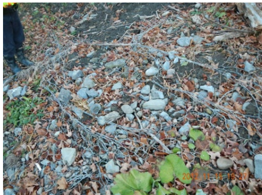
Photo 32: Erosion Site #3 along Reach TC-3
