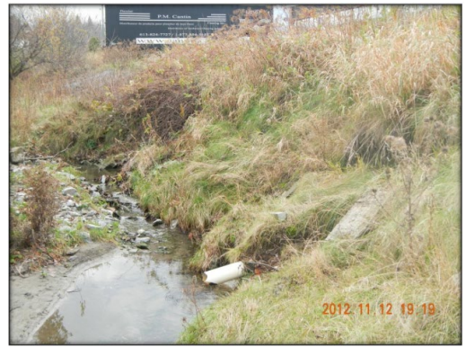
Photo 24: Erosion site #6 along Reach VC-2
