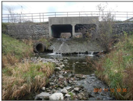
Photo 23: Erosion site #1 along Reach VC-2
