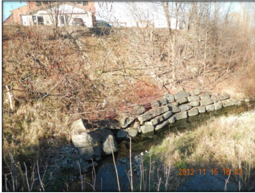
Photo 21: Erosion site #1 along Reach TC-3
