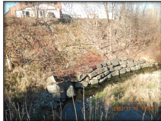
Photo 12: Priority Erosion Site within Taylor Creek, Undercut Armourstone Wall and Steep Valley Slope.
