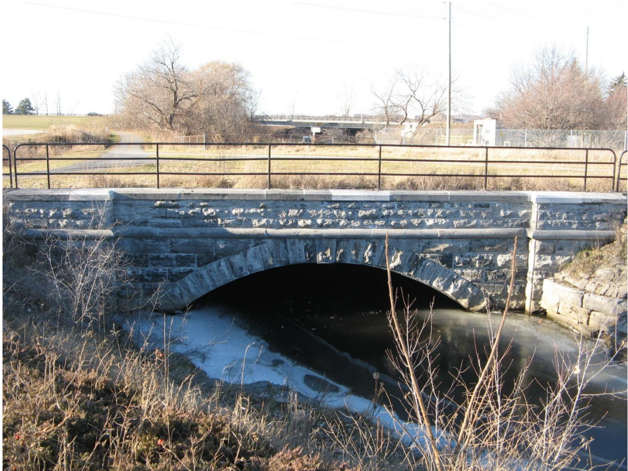
Figure 7: Former Central Canada Railway Bridge constructed in 1873 at the west end of the aqueduct, 2012. Only the east side of the bridge is visible; the rest of the bridge and a large portion of the aqueduct was covered for railway purposes early in its history. Source: https://s3.amazonaws.com/gs-waymarking-images/68e82f51-1ab6-4d55-90ec-ca61d0b7db4e.JPG .
