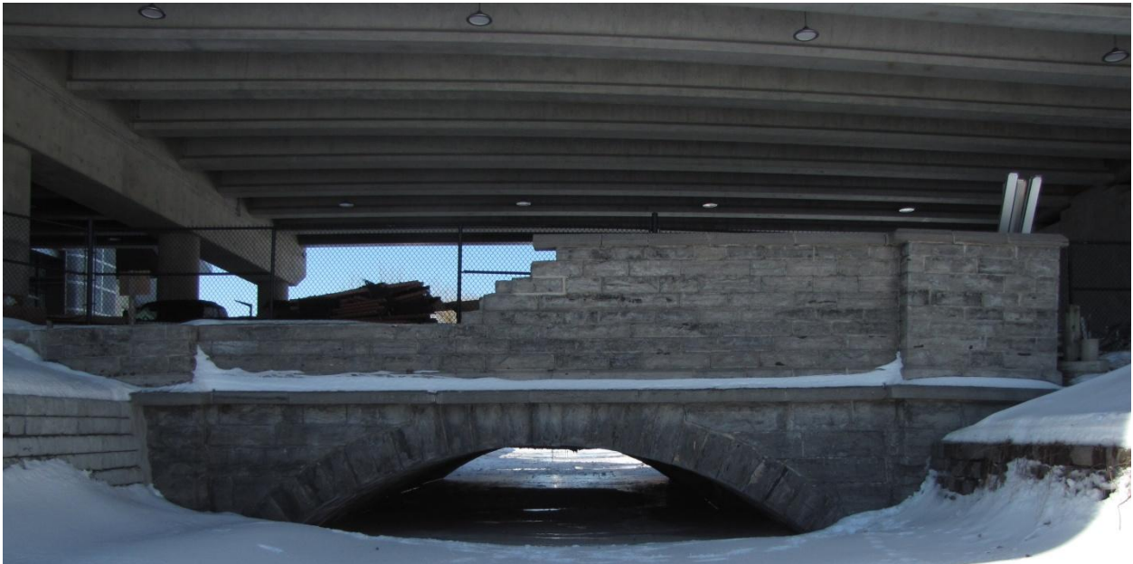
Figure 2: East arch and parapet of the Old Booth Street Bridge, March 2019. Source: Parsons.
