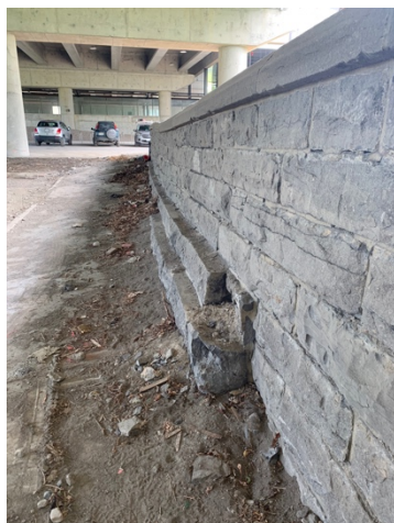
Figure 11: View of the west parapet wall of the West Extension looking south, 2019
