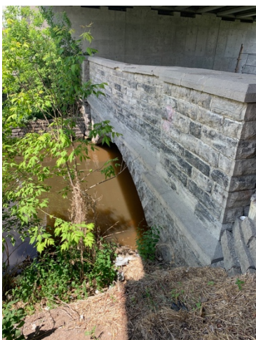
Figure 10: View of the west parapet wall of the West Extension looking north, 2019
