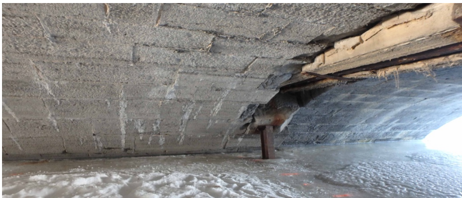
Figure 9: View of the existing watermain between the Centre Arch and the East Extension, 2018
