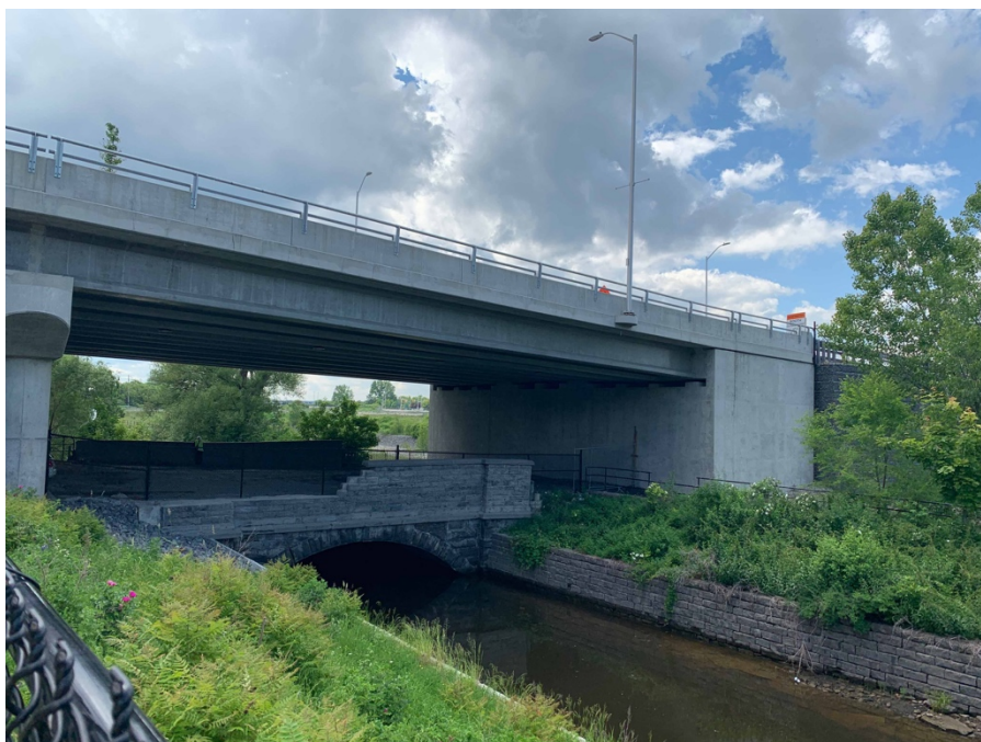
Figure 5: Photo looking northwest towards the Old Booth Street Bridge below the overhead Booth Street Bridge structure, 2019
