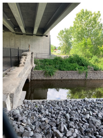
Figure 12: View of the east parapet wall of the East Extension dismantled in 2016, 2019
