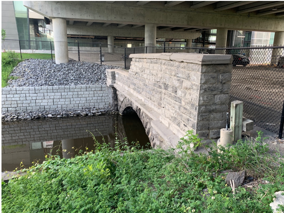
Figure 1: Overall view of the east side of the Old Booth Street Bridge, looking south.
