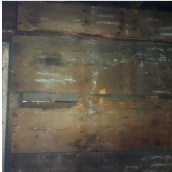
Photo Two – Dry Rot on Wood Framing
