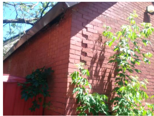
Photo Six – Significant Brick Bulging
