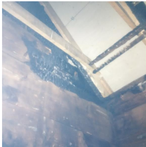
Photo One – Fire Damaged Roof Framing
