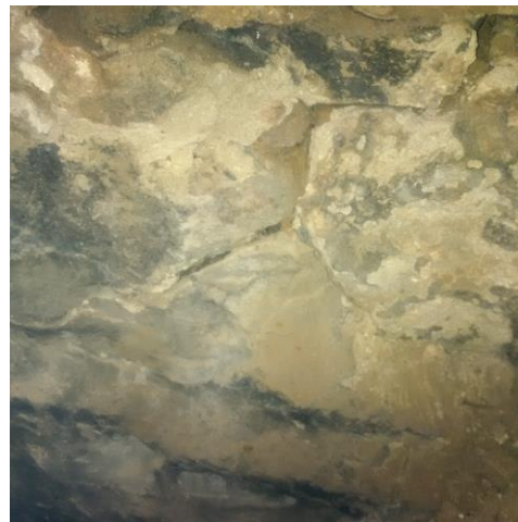
Photo Four – Deteriorated Mortar
