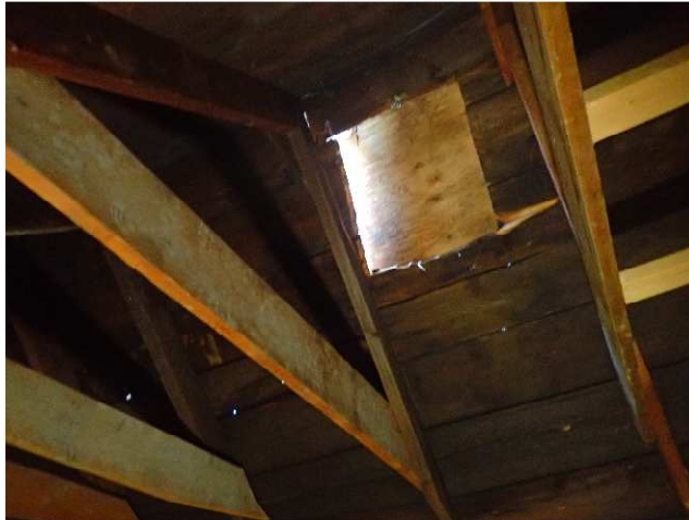
Photograph 7 – Daylight seen through holes in rear addition roof, JCAL (2016)
