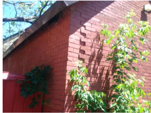
Photo Six – Significant Brick Bulging
