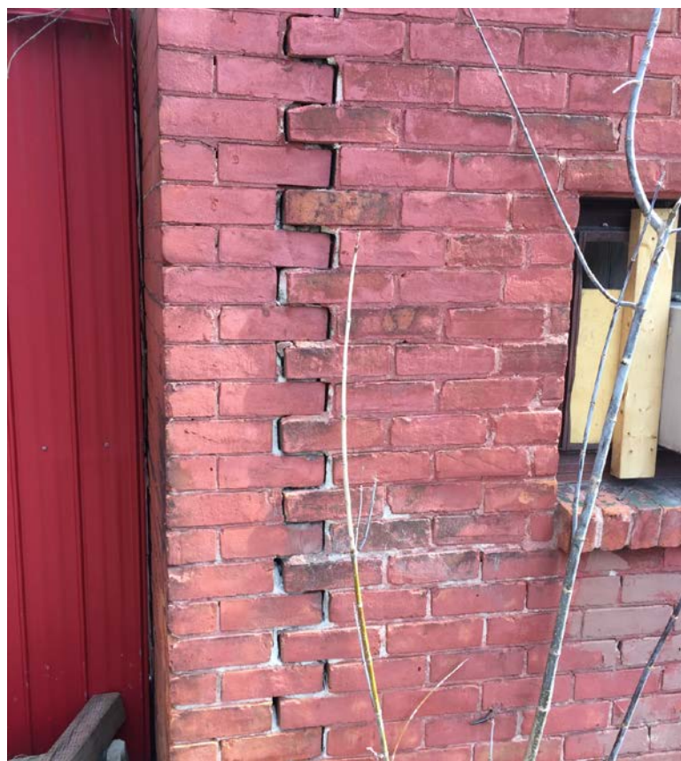
Figure 8: View of the west wall of rear wing illustrating the detached brick veneer.
