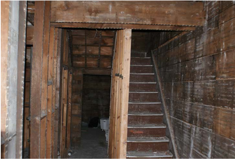
Figure 2: View of the interior stair. Note the horizontal board sheathing applied to the interior walls.
