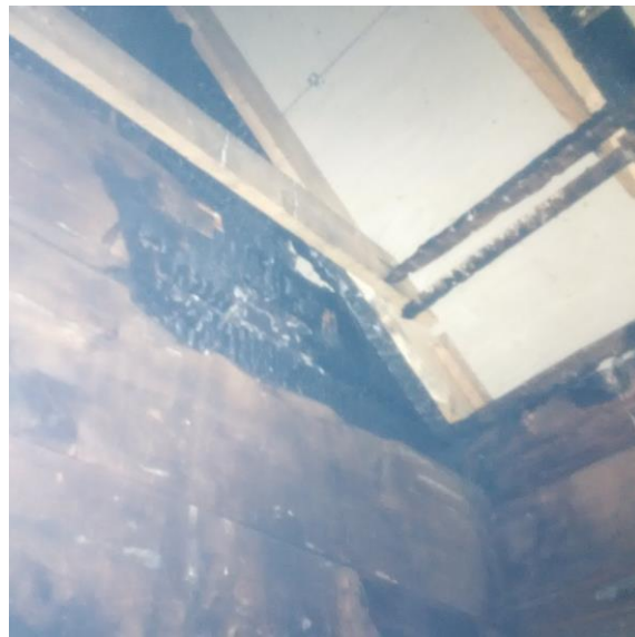
Photo One – Fire Damaged Roof Framing
