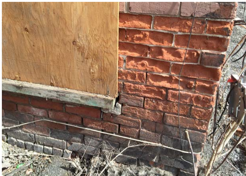
Figure 7: View of deteriorated brick at the base of the wall at the south-west corner of the front half of the building. Note the raised grade above the level of the stone foundation, and the buried brick headers at the top of a basement window.
