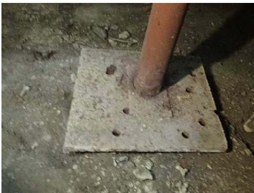
Photograph 6 – Steel tele-post bearing on soil, JCAL (2016)
