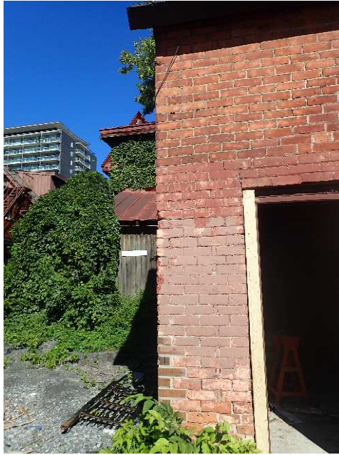
Photograph 9 - Step cracking above opening in west end of south wall, JCAL (2016)
