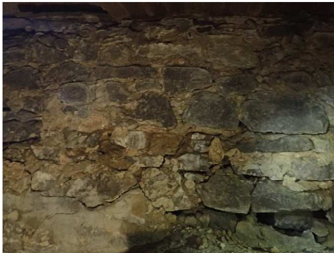
Photograph 1 – North wall with void joints, JCAL (2016)
