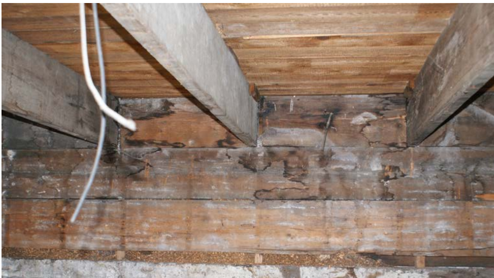
Figure 4: View of the balloon frame construction with second floor joists in the rear wing supported on 2" x 4" studs which are visible at the bottom of the photograph.
