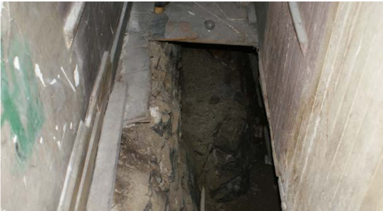
Figure 5: View down the stair to the basement. Note the displaced foundation wall which has been pushed into the building and the floor boards which have rotated upward.
