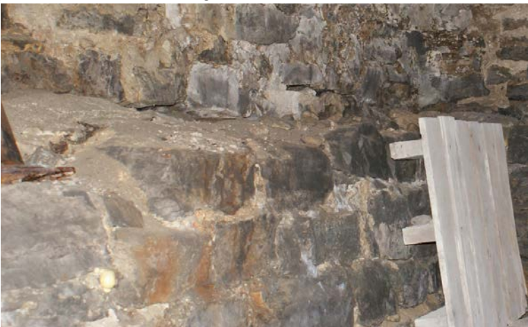
Figure 6: View of the foundation wall in the basement. Note the secondary stone wall at the base of the upper wall. This is a typical condition for foundation walls in front half of the building.
