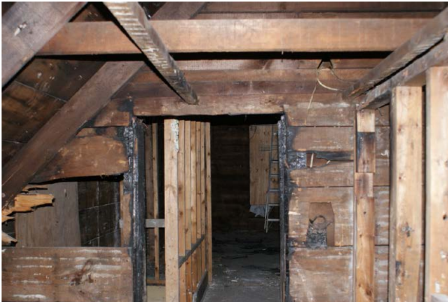
Figure 1: View from the second floor to the rear wing of the building where the fire would appear to have started.
