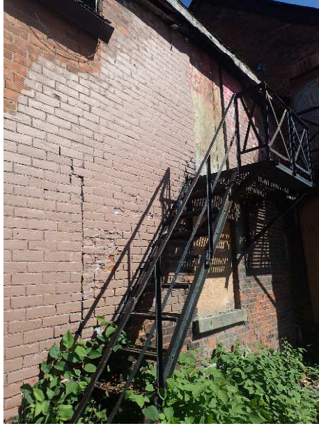
Photograph 5 - Break in running bond pattern between rear additions and spalling of painted brick, JCAL (2016)
