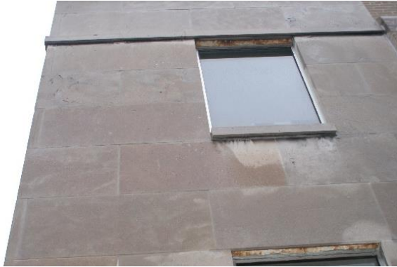
Figure 14: Note the rusting steel angle below the parapet belt course and the first floor window. There are indications on the north façade that the shelf angle below the parapet belt course is continuous. If this is the case, there is a high probability that the steel angle is secured to steel buried behind the wall.
