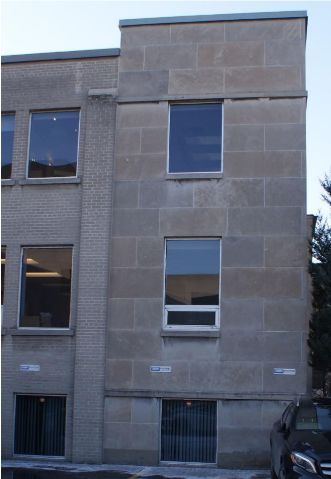
Figure 15: View of the east façade of the building. Note the lintel stone above the first floor window that overlaps onto the adjacent stones indicating a traditional load-bearing application. Note the projecting brick pilaster and its termination at the top. A steel column is likely buried behind the pilaster. The beam may support additional horizontal steel beams that would support the parapet, to which the continuous shelf angle evident below the parapet belt course would be attached.
