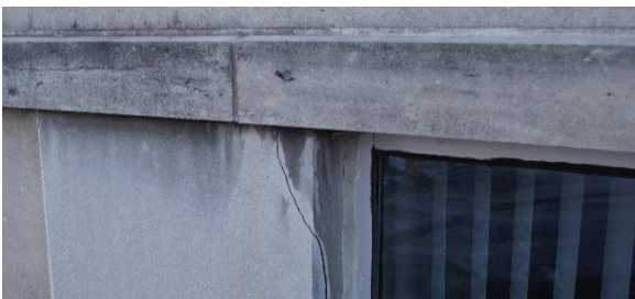
Figure 10: View of a stone in the belt course (left) that has different material characteristics in the process of fracturing at a bedding plane. Source: CHRM.
