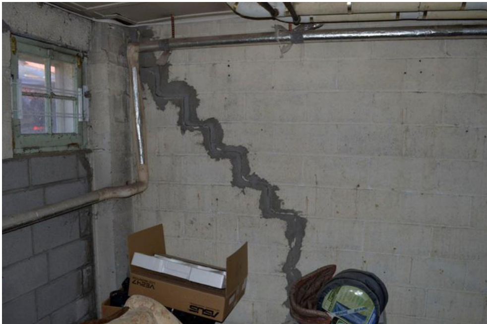
Cracking in foundation wall
