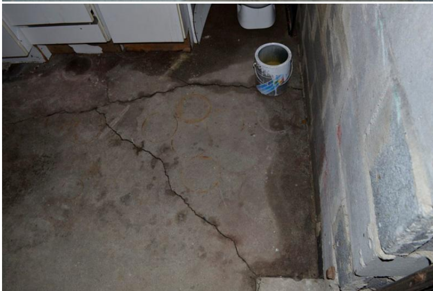
Cracks in floor slab
