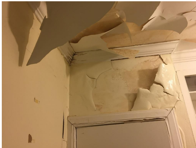
Photo 9: Severity of plaster and paint issues in kitchen effectively hide structural cracks. However, a number of cracks were noted including the doorframe visible in this photo.
