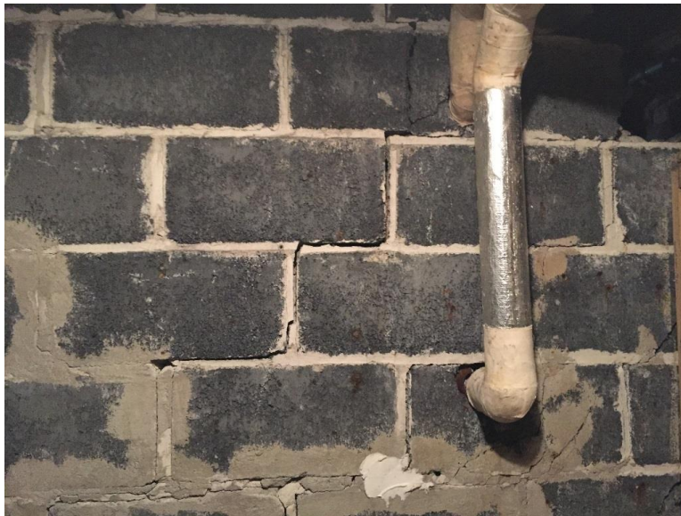
Photo 4: Block masonry walls in basement show multiple repairs and ongoing step cracking in numerous locations (typical).
