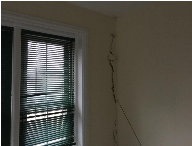
Photo 11: Similar to noted issue on level 1, some of the most severe wall cracking noted along south elevation (office - 209).
