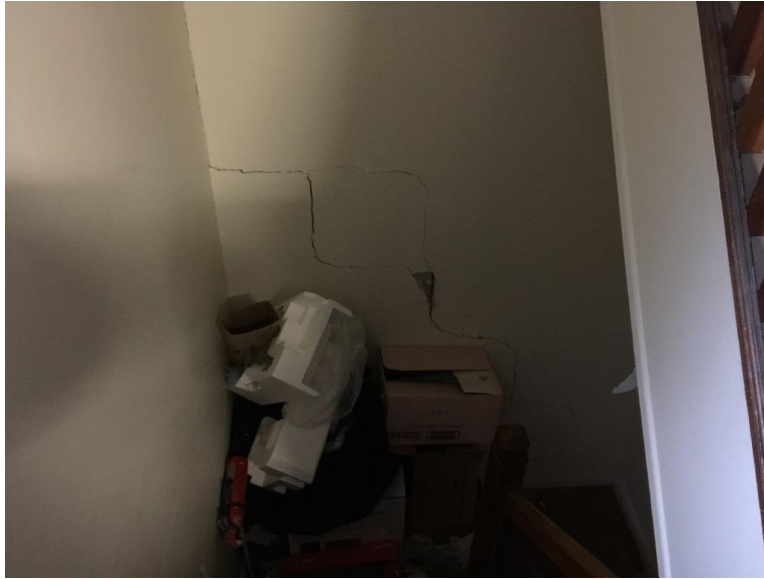
Photo 13: Step crack in stairway along east elevation.
