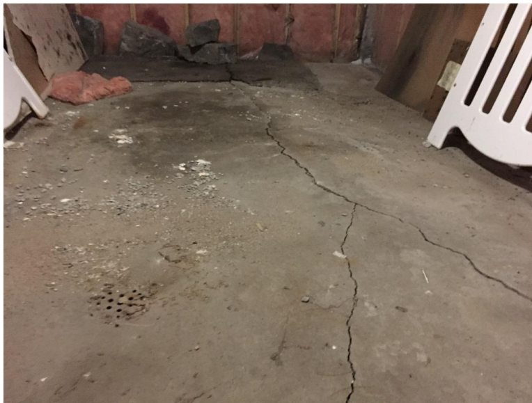
Photo 2: Extensive slab on grade cracking in former garage along northwest area of basement.
