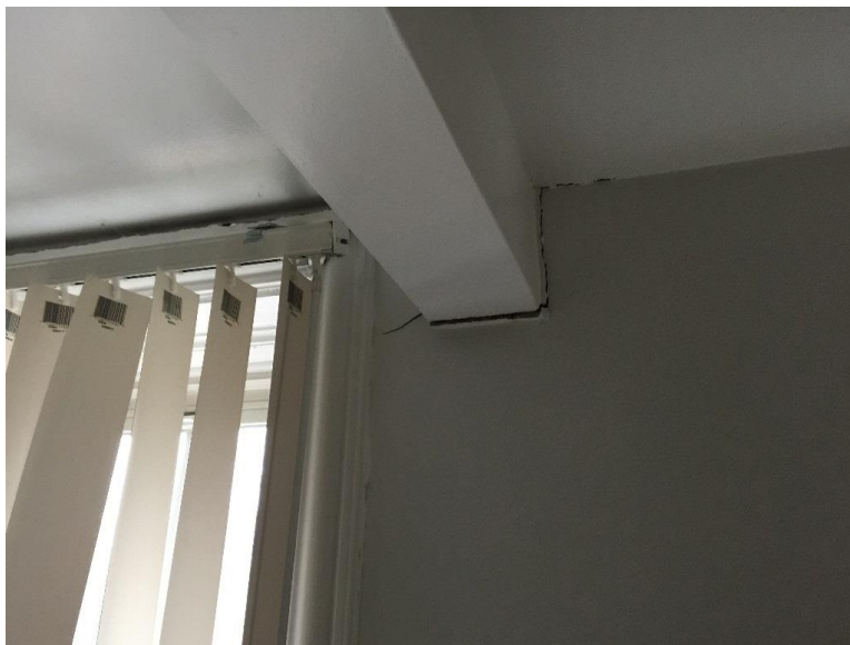
Photo 14: Significant movement indicated by pattern of cracks noted along north elevation at end of corridor.
