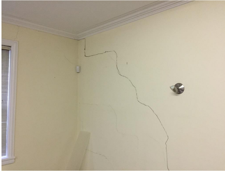
Photo 17: Extended crack at interior wall along west elevation in High Commissioners Office - 210. Although not clear in photograph, multiple separate horizontal cracks exist at roughly 3 ft. intervals down the wall.
