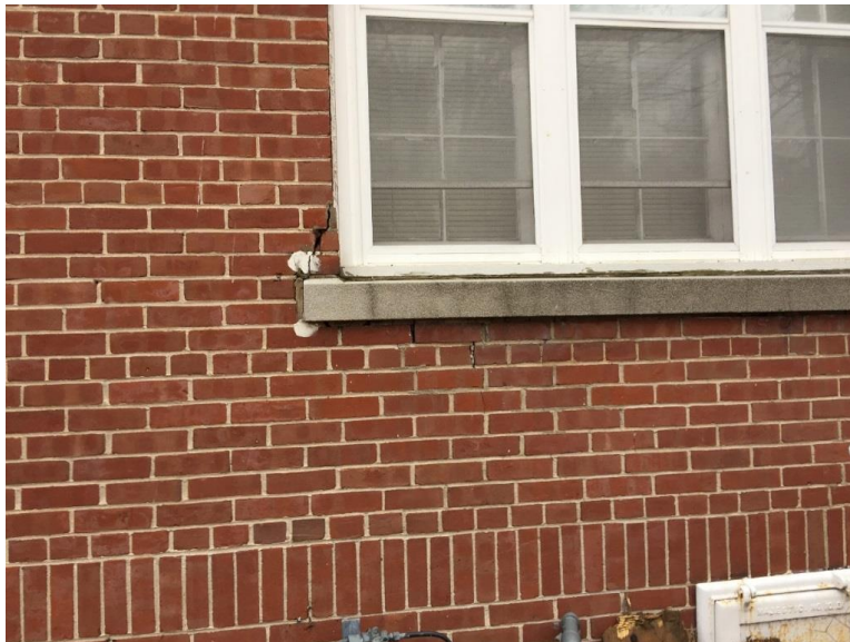
Photo 19: This large crack and step cracking beneath window sill on south elevation indicative of conditions throughout the building.
