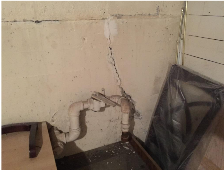
Photo 3: Cracking of poured in place concrete basement wall in the southeast corner of the building.
