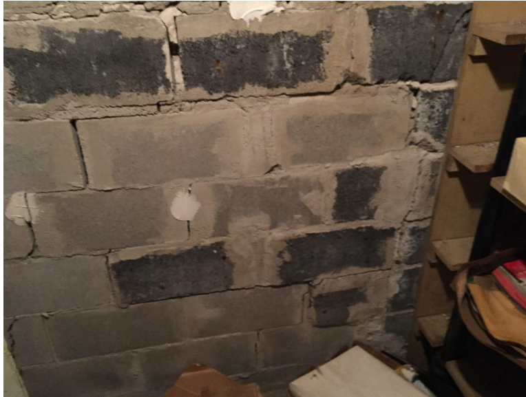
Photo 5: This location shows one of numerous repairs with ongoing step cracking (typical).
