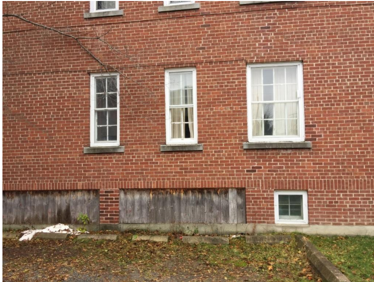
Photo 18: The exterior brick cladding shows multiple repairs.
