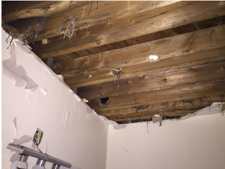
Photo 10: Failure of ceiling likely the result of ongoing water damage.
