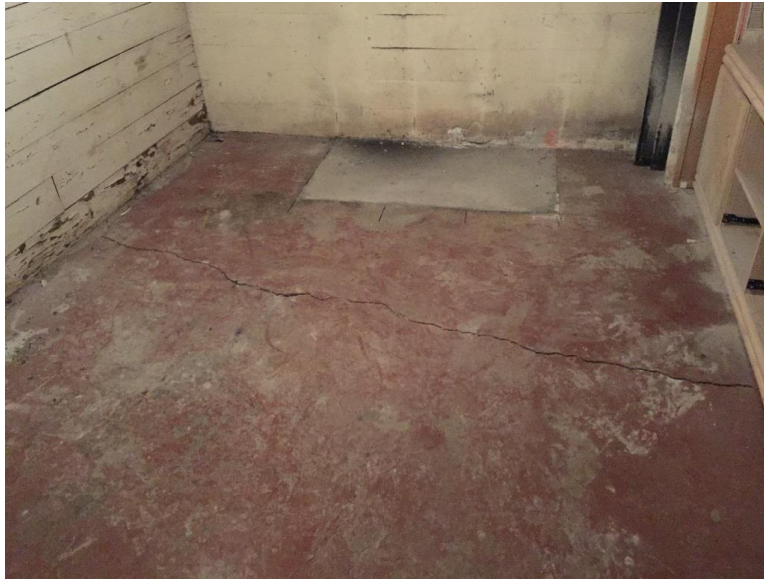
Photo 1: Crack in slab on grade noted basement utility room at southeast portion of the building.
