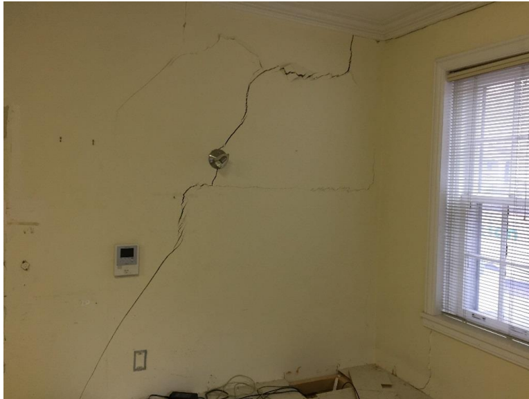
Photo 6: Extensive crack on interior wall along south elevation (Living Room - 113).
