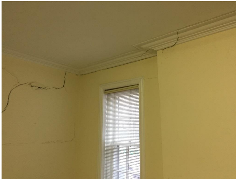
Photo 7: Cracking shown in photograph 6 continues along south wall.
