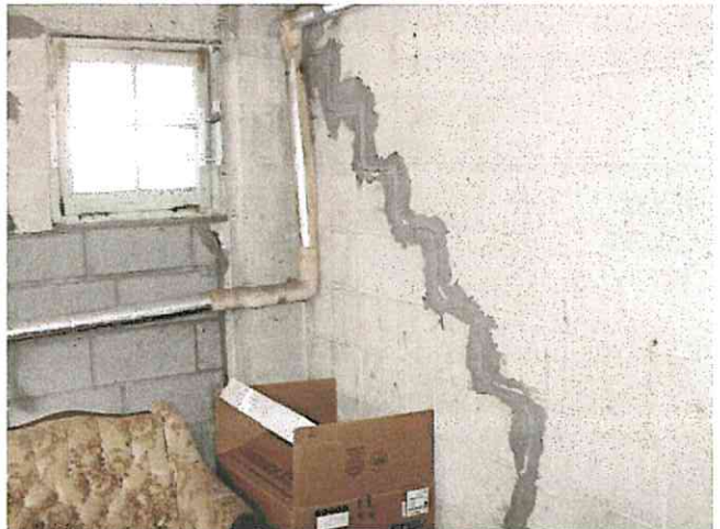
Photo 2 - Showing an example of a crack in a load bearing wall.
