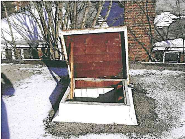
Photo 7 - Showing an unsecured roof hatch as well as corrosion on roof hatch.
