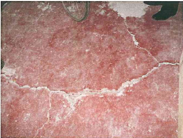
Photo 3 - Showing an example of a crack in the slab-on-grade.
