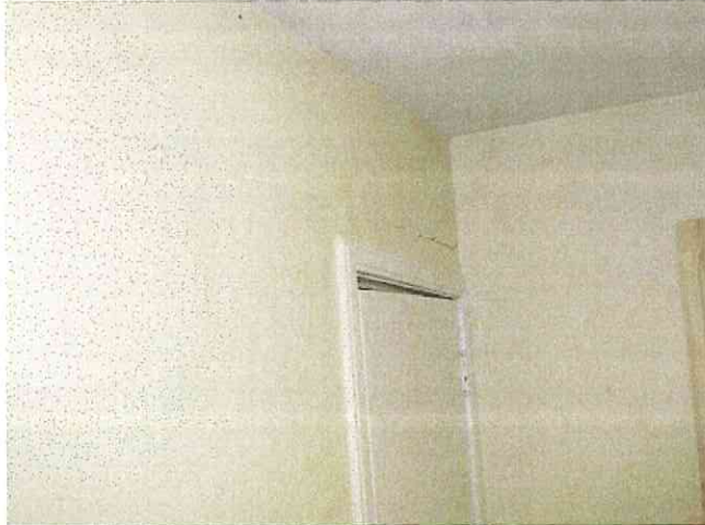
Photo 5 - Showing an example of an off-level door within the door frame, and also showing an interior drywall crack.
