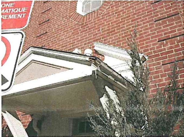
Photo 9 - Showing deteriorated wood deck at canopy roof.
