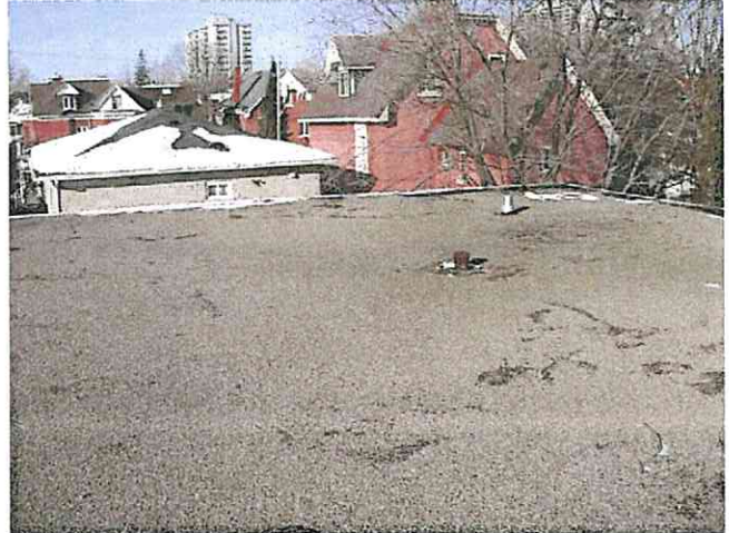
Photo 6 - Showing isolated exposed flood coat due to scoured gravel ballast, and also showing a corroded roof drain.
