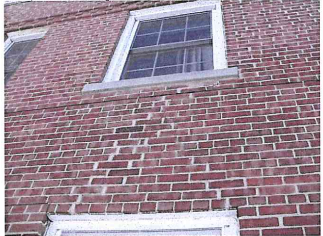
Photo 8 - Showing typical cracked mortar joints in solid brick masonry between windows.
