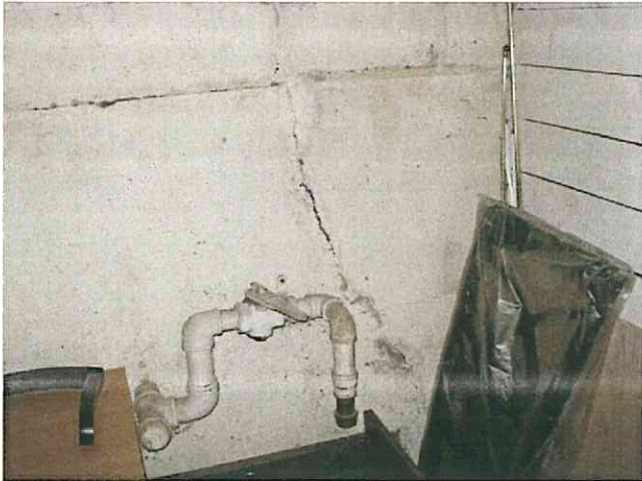
Photo 1 - Showing an example of a crack in the foundation wall.
