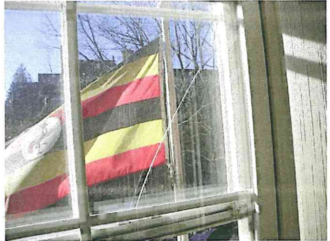
Photo 10 - Showing a cracked window pane.
