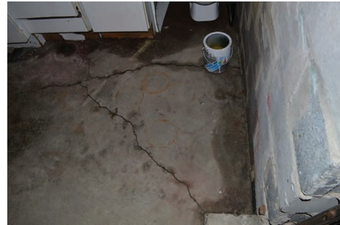
Cracked basement slab and water infiltration.
