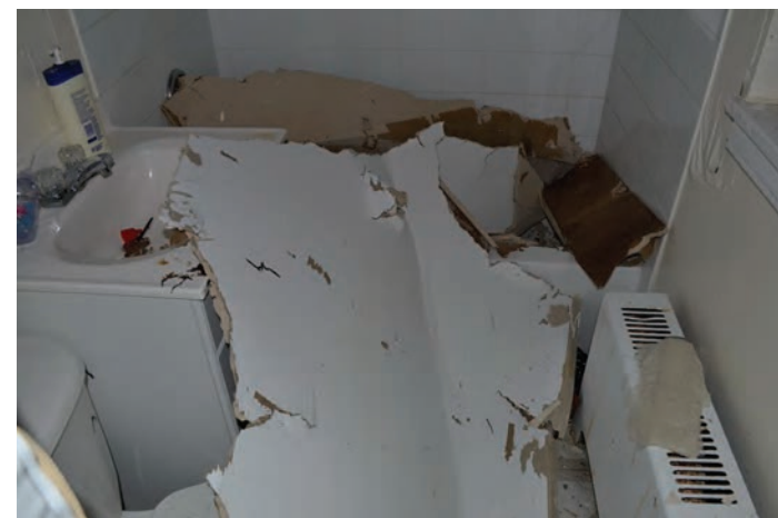
Collapsed drywall ceiling due to water infiltration.
