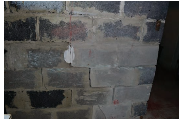
History of crack repairs at basement foundation wall indicates ongoing problem of settlement. Note the concrete block replacements.
