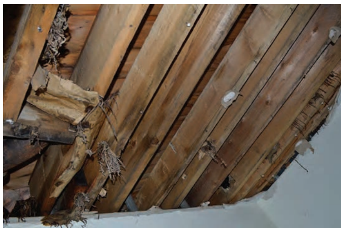
Exposed floor joists at collapsed drywall ceiling due to water infiltration.
