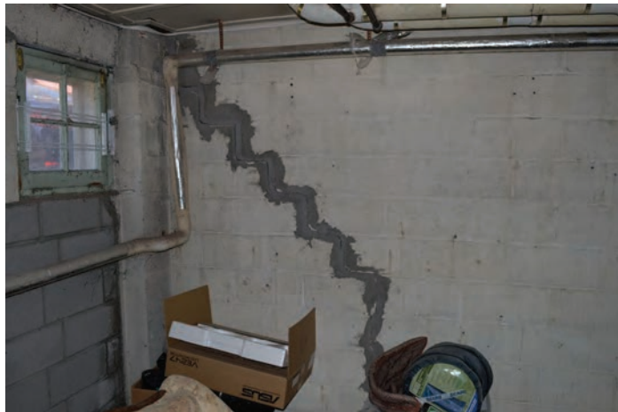
Evidence of repairs at extensive cracking in basement foundation wall.
