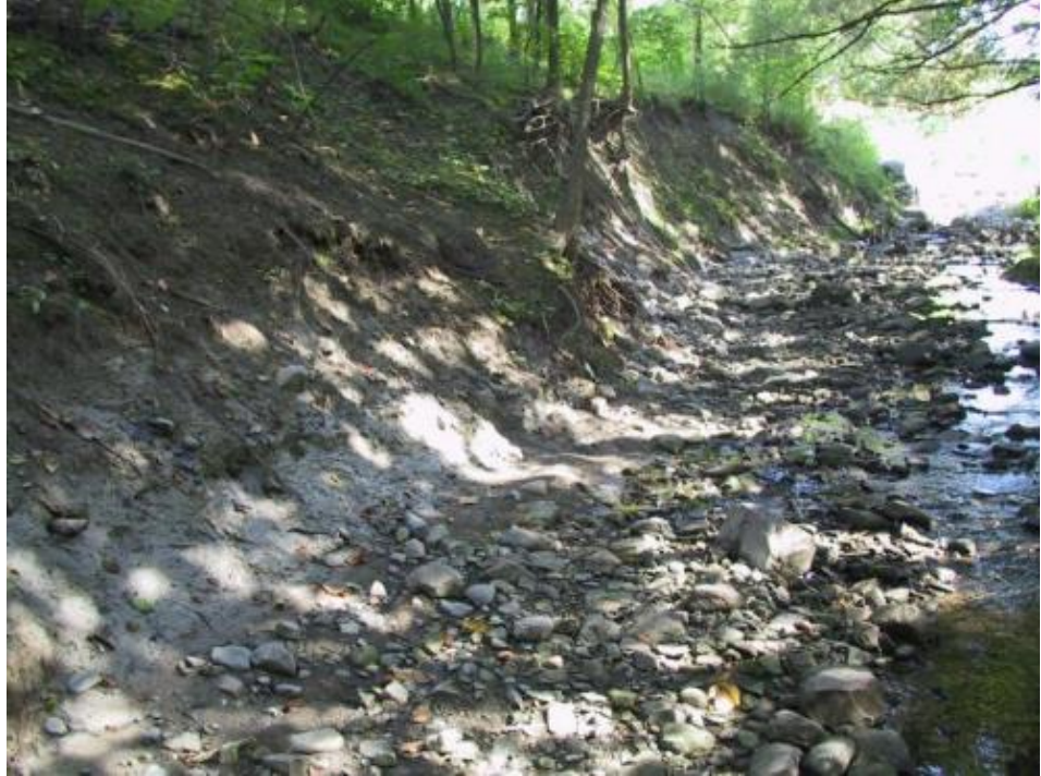
Photo 1: Eroding east bank downstream of gabion wall (Reach 6). View is looking upstream (JFSA, 2015)
