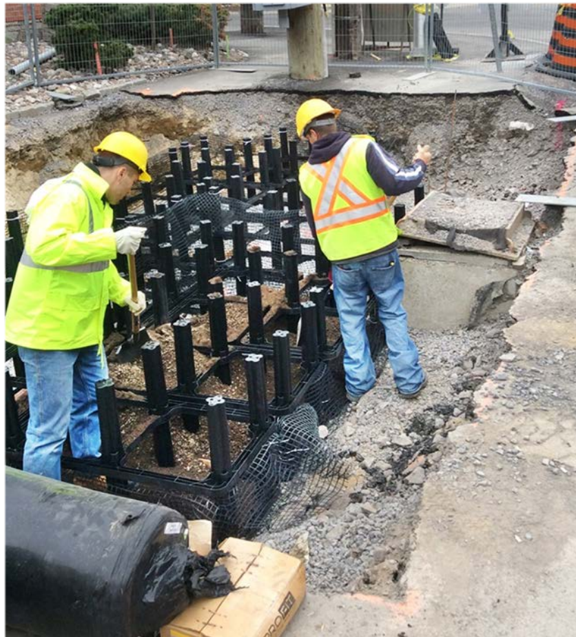
Figure 10: Installation of Silva Cell structural soil cells to provide adequate soil volume for trees along Gladstone Avenue. Image source: Douglas Associates Landscape Architects, 2015 (drcla.ca).
