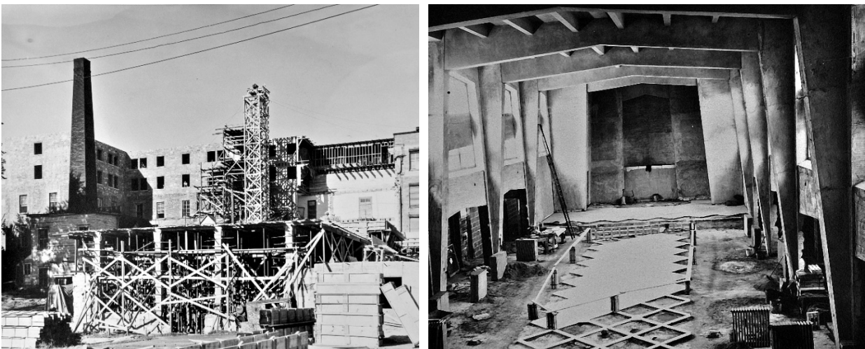
Views of the chapel under construction. Supposedly, the construction crew included priests using the novitiates and lay members of the order as the labour force.
