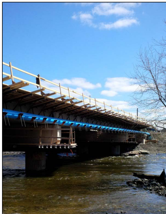
Figure 11: Watermain on Bridge
