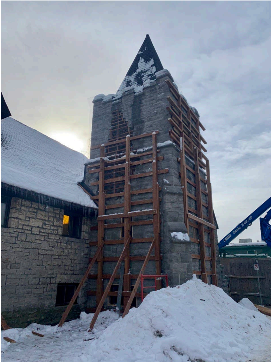
Photo of the west/north sides of the tower showing the completed bracing and cracking. Photo taken January 2021
