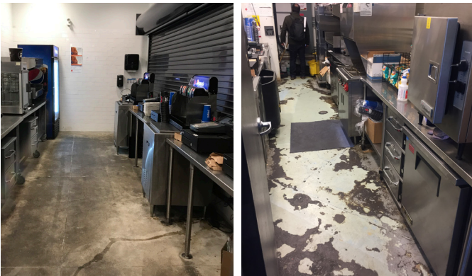
Condition of concession and lack of grease hood
