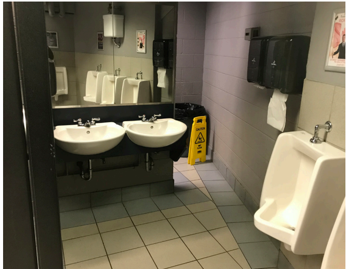
Inadequate lavatory count/clearance/accessibility
