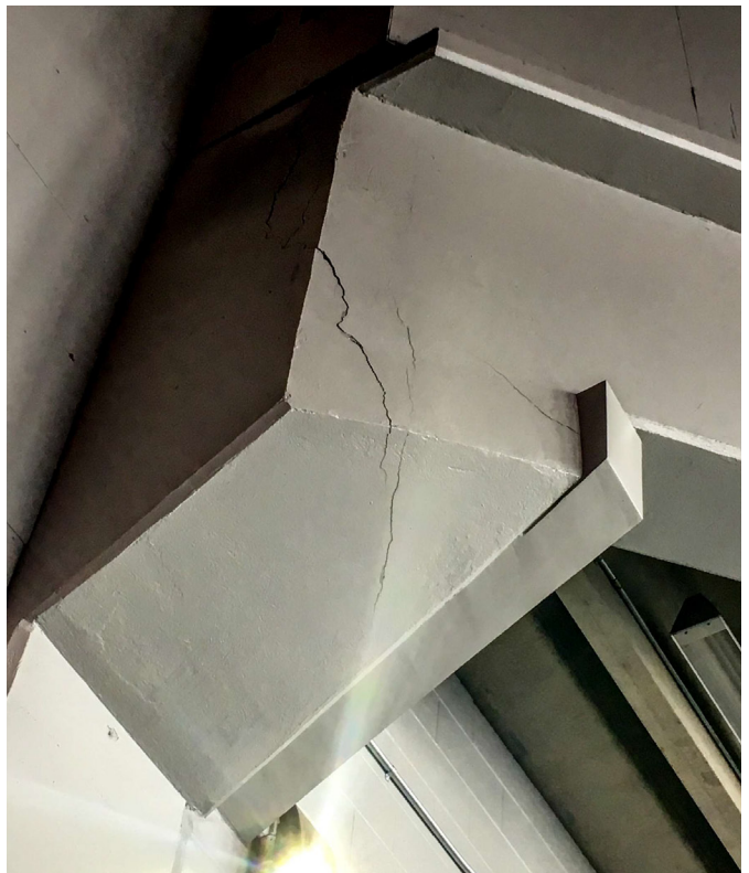
Structural concrete damage - investigation recommended
