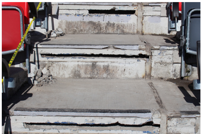
Deteriorating stadia/joint condition
