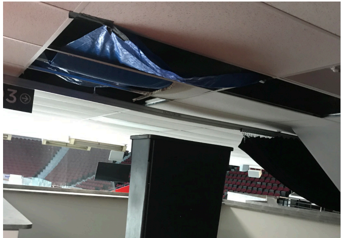
Water damaged ceiling tiles at lower concourse.
