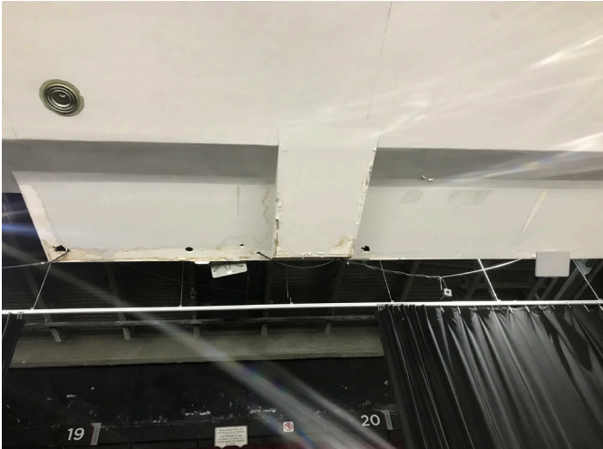
Severe water infiltration causing mold/damage
