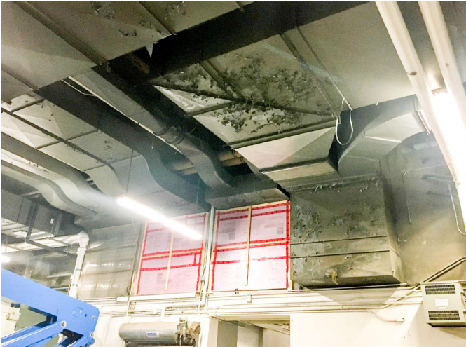
Severe water infiltration causing mold/damage
