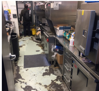
Concession conditions/ no grease duct capability
