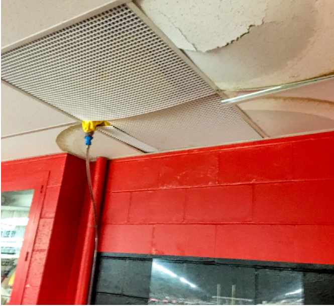
Severe, repeated water damage at lower concourse
