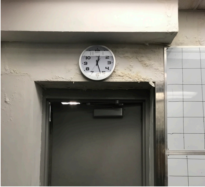
Severe water infiltration causing mold/damage
