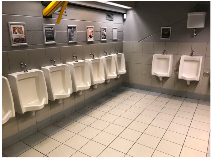
Improper spacing, lack of urinal screen, low head clearance
