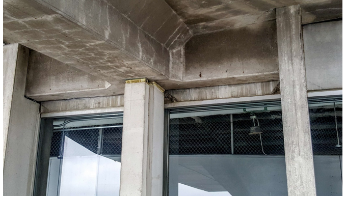
Water seepage and efflorescence
