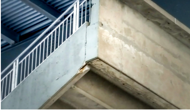
Spalling concrete exposing steel reinforcing
