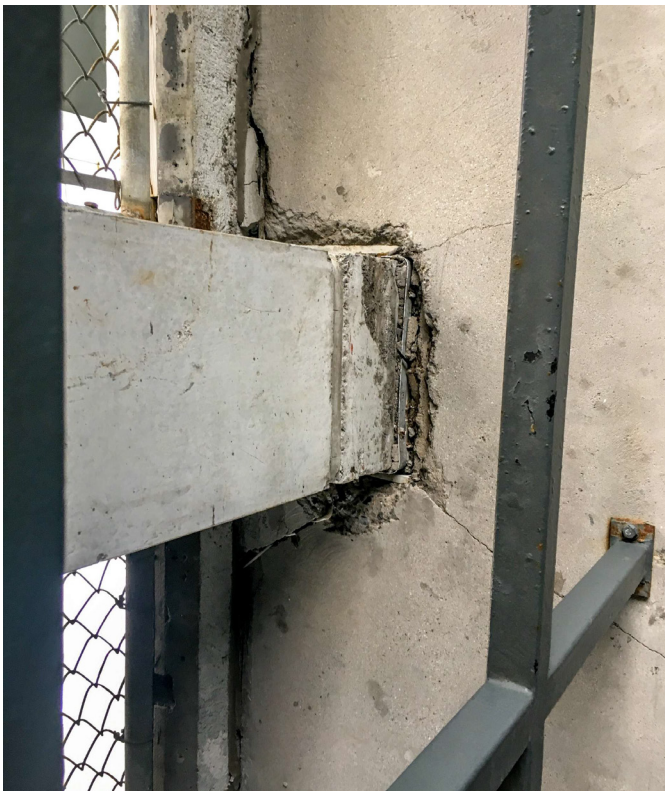
Severe concrete cracking/slab damage
