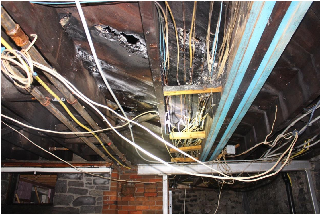
Photograph 9: View of drop down charring of the ground-floor framing.
