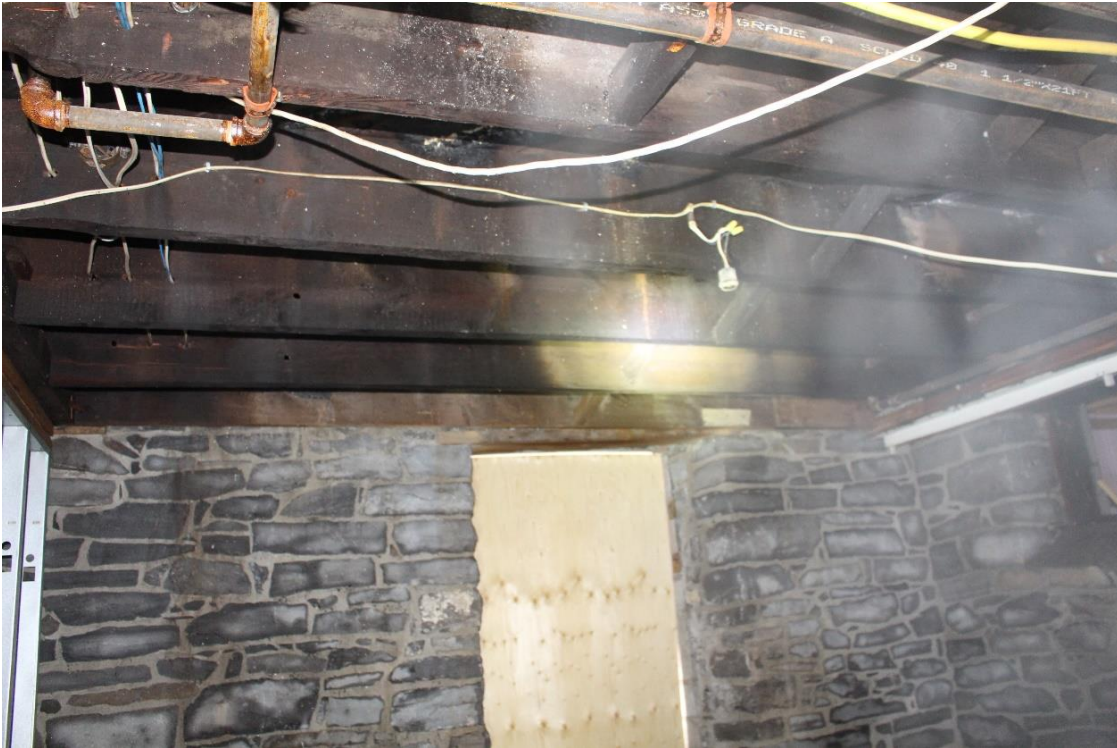
Photograph 10: View of smoke staining in the basement.
