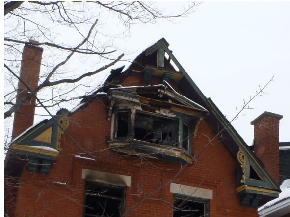
Figure 9: Damaged bargeboards on south gable [JCAL 2021]
