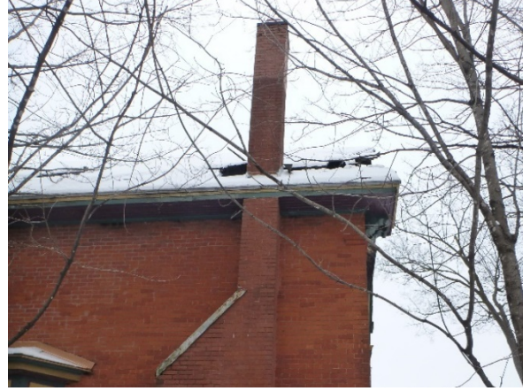
Figure 7: Laterally unsupported west chimney at large hole in roof [JCAL 2021]
