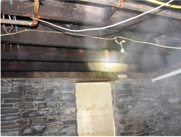
Figure 4: Smoke-stained basement joists [DFA 2021]
