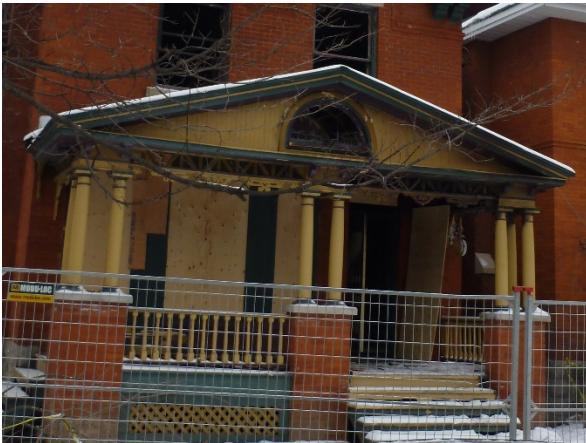
Figure 8: Front porch, smoke-stained spandrel [JCAL 2021]
