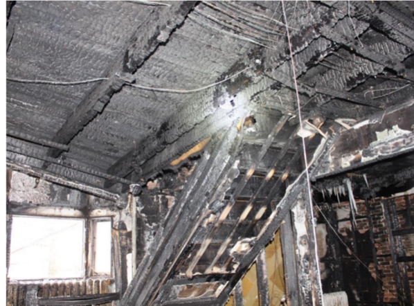
Figure 5: Charred and deflecting second floor joists [DFA 2021]
